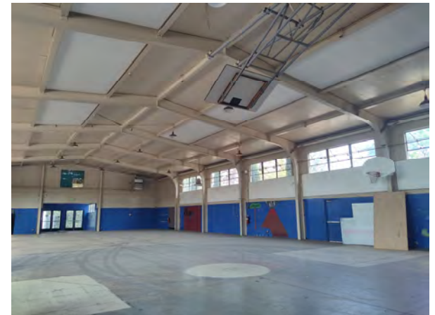
Photo 3. Interior of main building facing northwest from southeast corner of main building (July 29, 2021).
