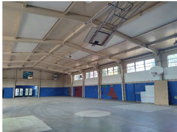
Photo 20. Interior of main building facing northwest from southeast corner of main building (July 29, 2021).
