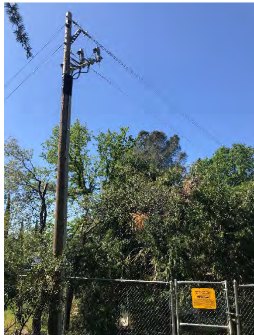
Photo 12. View of an electrical pole without transformers in the central portion of the Site (March 2022).
