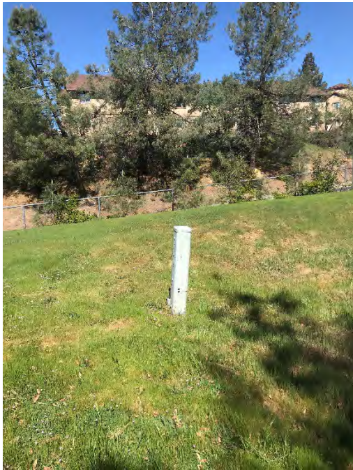
Photo 7. View of electrical facilities in eastern-central portion of the Site (March 2022).
