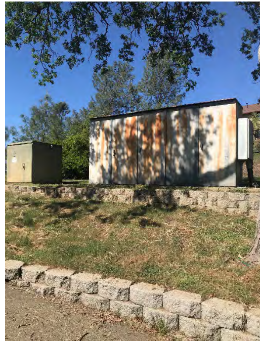
Photo 8. View to the west of electrical facilities in the northeastern portion of the Site (March 2022).
