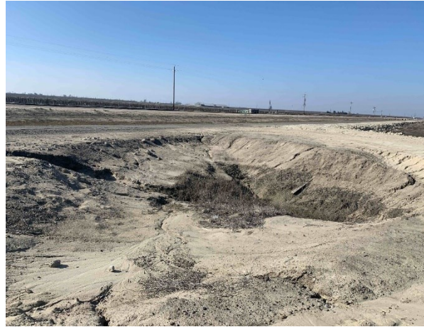
Photograph 4. View of sedimented culvert at southeastern corner of the project site, facing southwest.
