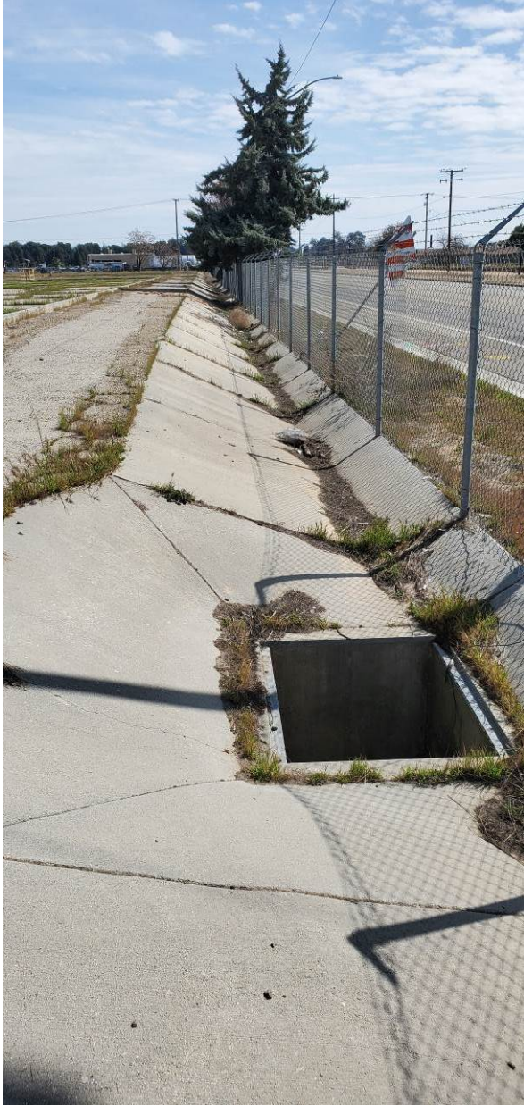
Photo 7: Onsite drainage ditch along southern side of site leading to drain inlet in foreground.
