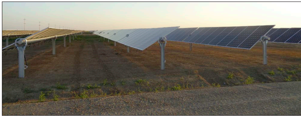
Solar PV Modules on Horizontal Trackers
