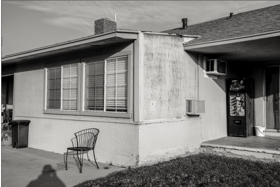
Photo 9: Enclosed Patio Porch. Note Loss of Fabric, Feeling, and Condition Noted in Photo 9. Note use of 2"x4" Studs, instead of Appropriate 1"x4" Common Board for Casing View Northwest. DSC7130
