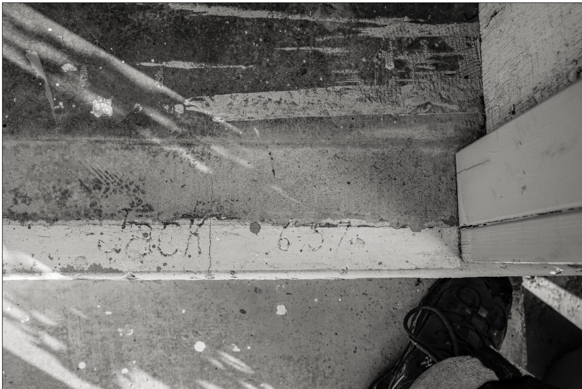
Photo 14: Date Stamp in Rear Patio Porch Slab. Note Removed Stem Wall Ghost Print in Modified Entryway
