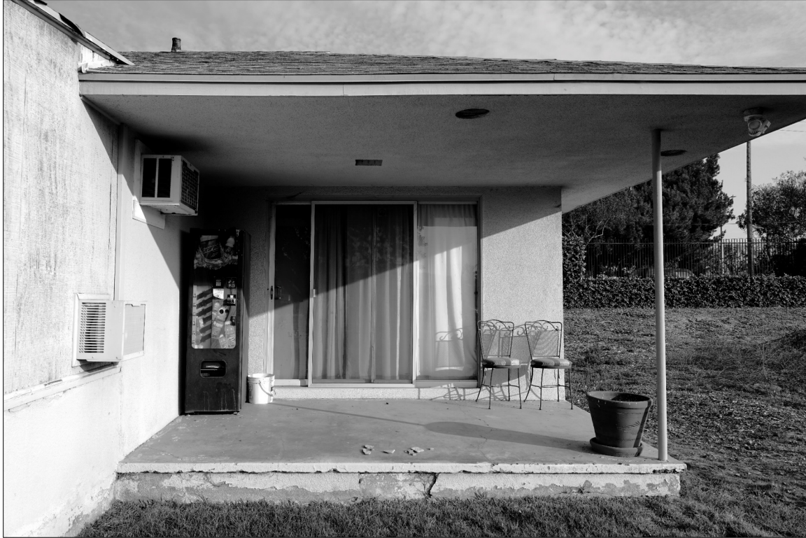
Photo 11: Patio at Southeast Corner of House with Original Aluminum Sliding Doors and Casework. Note Rough-Sawn No Bead Plywood Siding Enclosing Patio Porch and Loss of Fabric Noted in Photo 9. View North
