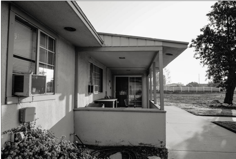
Photo 8: Rear Patio Porch with Original Finishes. Note Vertical Drop-Lap Siding below Shed Roof, and Original Framing. Note Replacement Vinyl Windows and Doors and 1"x4" Casement. Note Round Soffit Vents. View East. DSC7121
