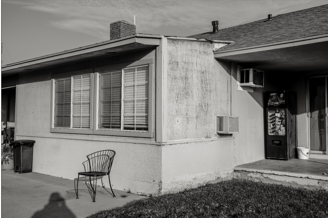
Photo 10: Enclosed Patio Porch. Note Loss of Fabric, Feeling, and Condition Noted in Photo 9. Note use of 2"x4" Studs, instead of Appropriate 1"x4" Common Board for Casing View Northwest
