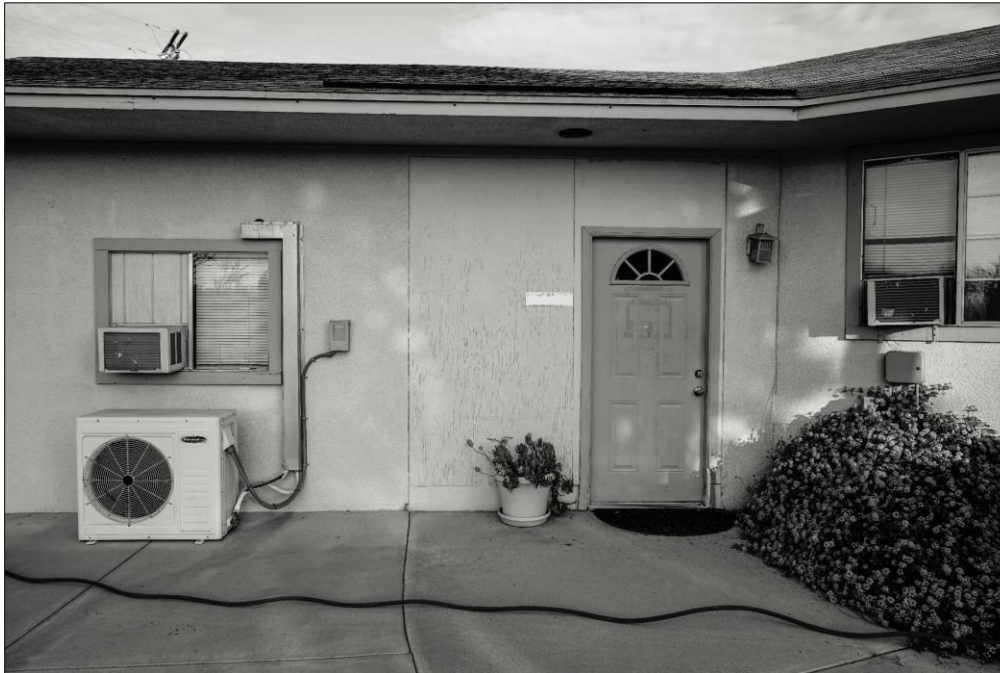
Photo 6: Low-cost Incompatible Infilling of Prior Aperture Between Main House (R) and Garage (L). View North. DSC7120
