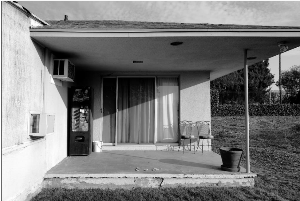
Photo 10: Patio at Southeast Corner of House with Original Aluminum Sliding Doors and Casework. Note Rough-Sawn No Bead Plywood Siding Enclosing Patio Porch and Loss of Fabric Noted in Photo 9. View North. DSC7142
