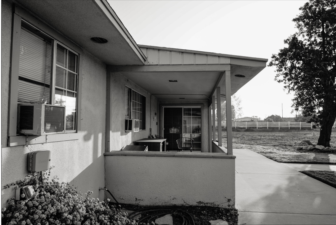
Photo 9: Rear Patio Porch with Original Finishes. Note Vertical Drop-Lap Siding below Shed Roof, and Original Framing. Note Replacement Vinyl Windows and Doors and 1"x4" Casement. Note Round Soffit Vents. View East
