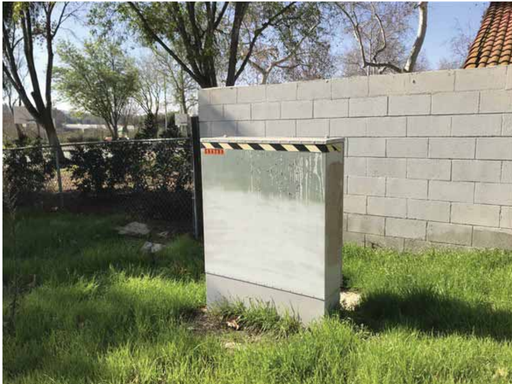
Photo 22: Western-facing view of a electrical panel or transformer located along the western side of Beltramo Road.
