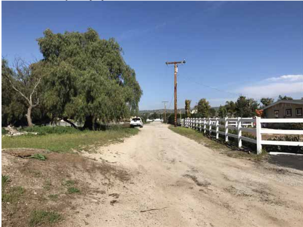
Photo 24: Northern-facing view along the unpaved southern portion of Beltramo Road; one of three pole-mounted transformers is also pictured.
