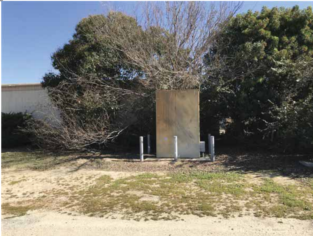
Photo 18: Eastern-facing view of a pad-mounted transformer that is located adjacent to the west of the modular-church-facility buildings.
