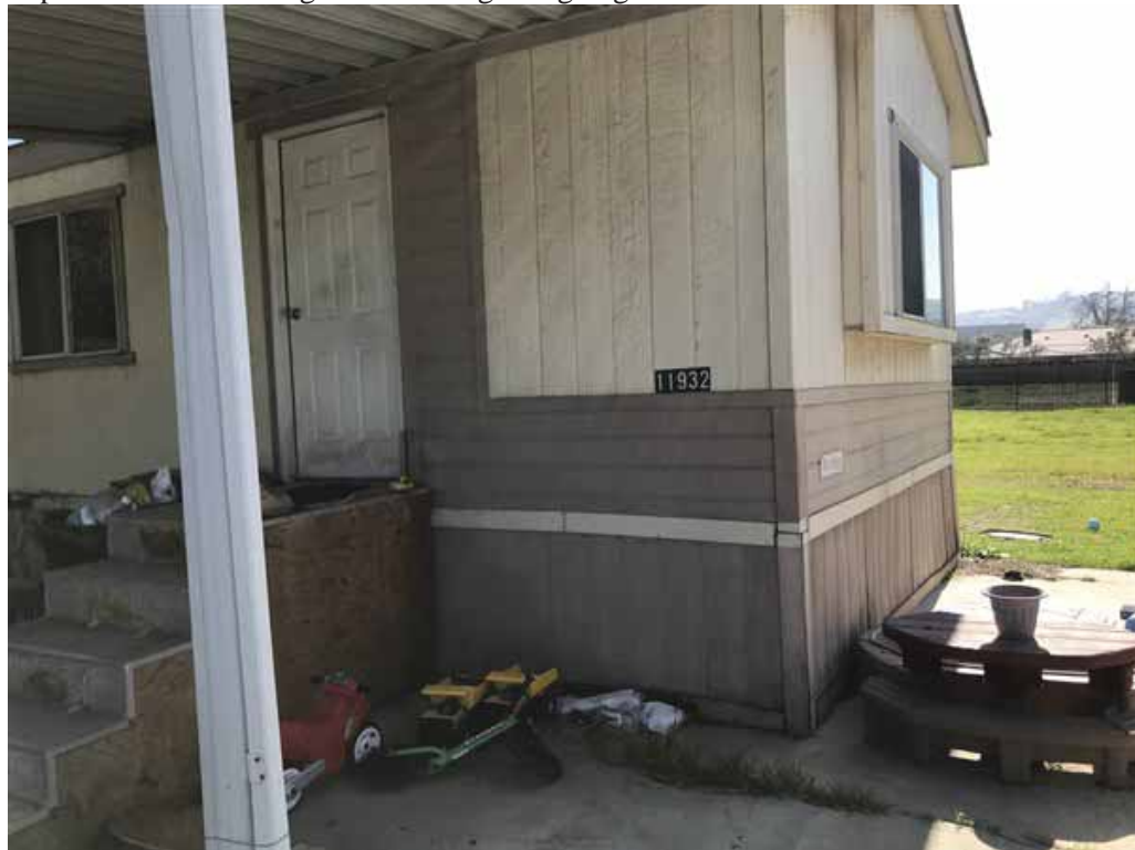
Photo 16: Close-up view of the Mobile Home located within Parcel 4 that depicts the address of 11932 E. Los Angeles Avenue.
