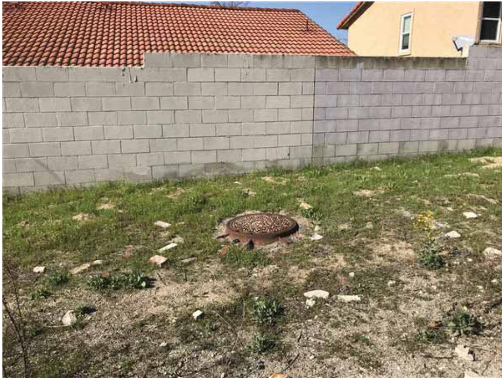
Photo 23: Western-facing view of what appears to be a stormwater manhole located on the west side of Beltramo Road. The adjacent properties to the west are residential.
