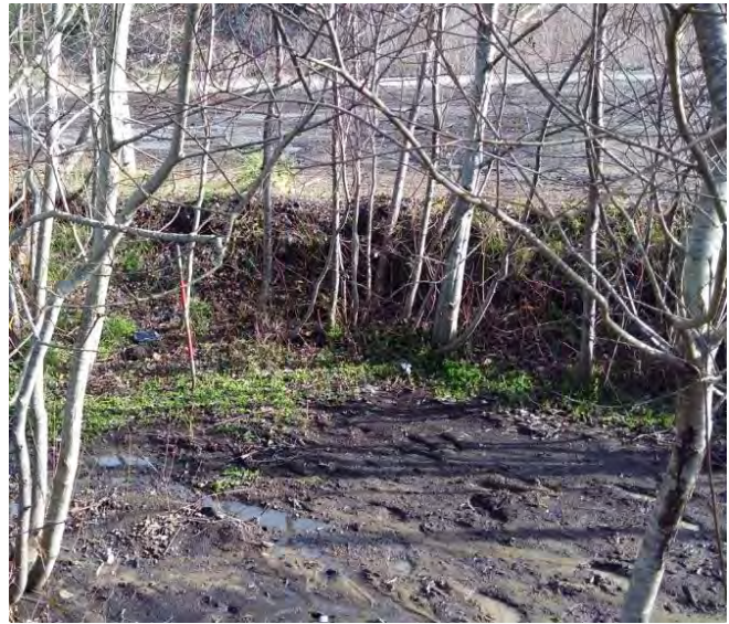
Photo B18: TP17U Site looking north. Note captured sediment and industrial use beyond. Sediment is removed annually.
