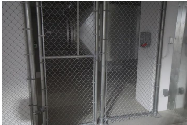
Typical ventilation fan enclosure in parking garage
