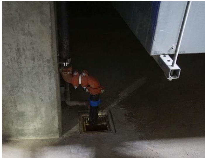
Floor water drain, NW corner of Floor P1
