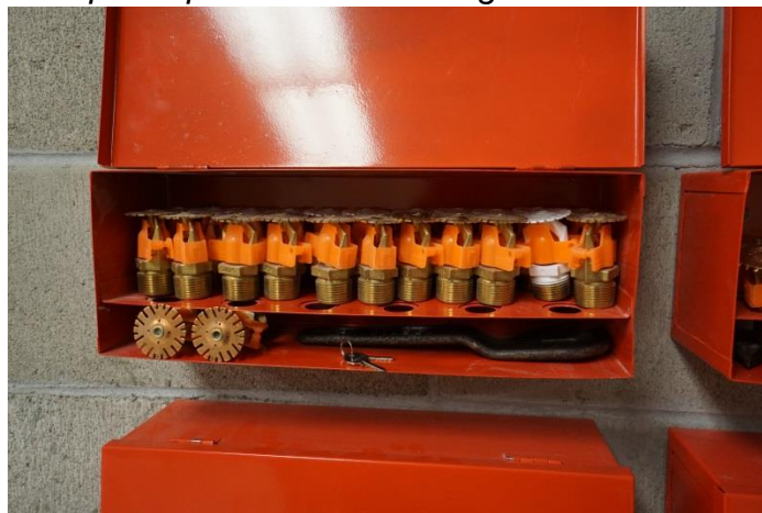
Some of the spare sprinkler head storage in the Fire Control Room
