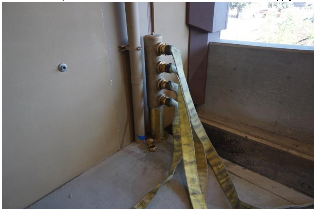
The Fire Department Connection with fire hose connected for supply
