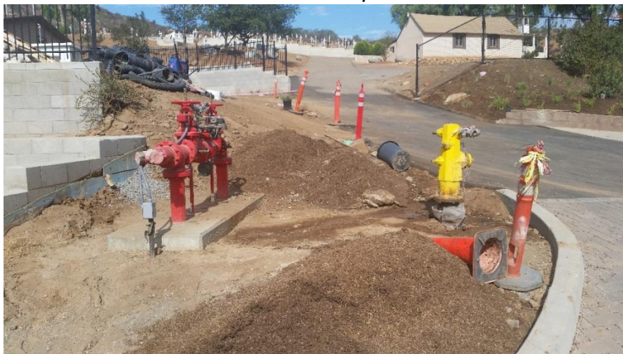
Wastewater treatment Fire Department Connection
