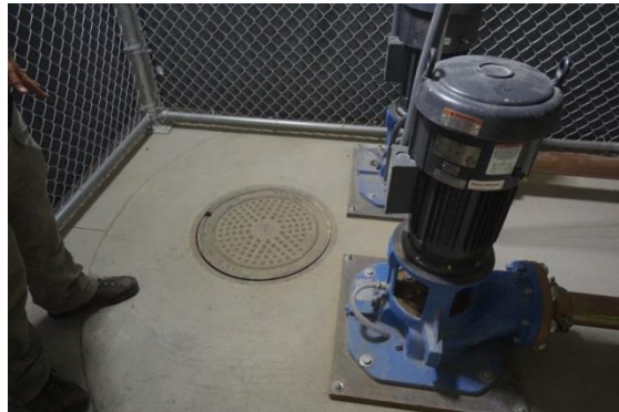
Sewer cover and sump pump - DO NOT USE FOR FIRE DRAINAGE
