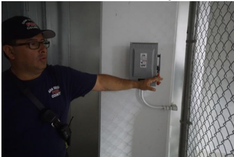
Turn on manual switch in exhaust fan cage to exhaust air
