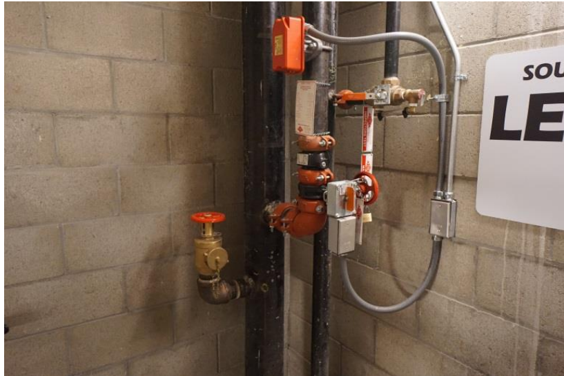
Typical stairwell standpipe connection (left) and fire sprinkler sectional valve (right)
