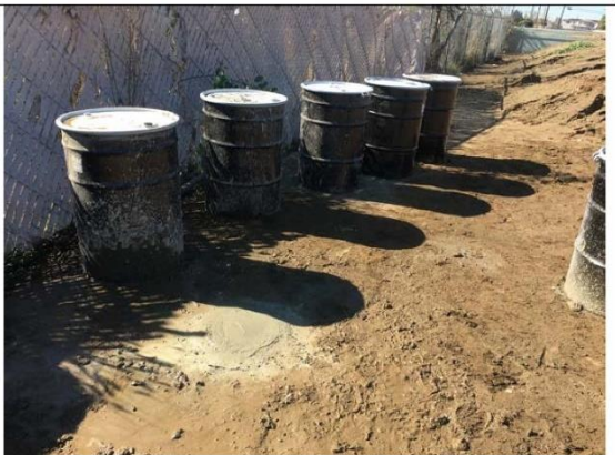
Photo 9. Finalization of abandoned well with cement and five 55-gallon waste soil drums.
