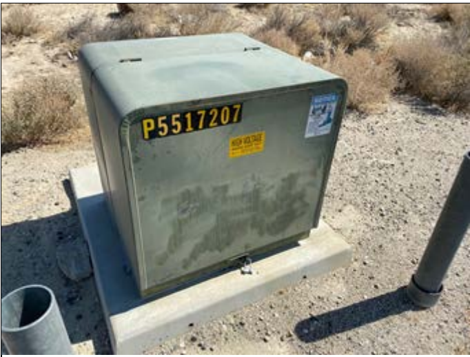
21. View of pad-mounted transformer
