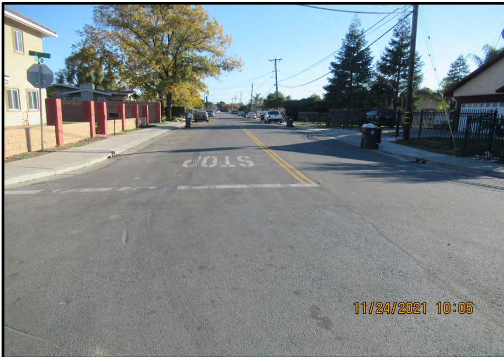
West end of the off-site storm drain line, looking east down 13th Street from B Street; 11/24/21. The storm drain line will tie in to the existing storm drain line in B Street.
