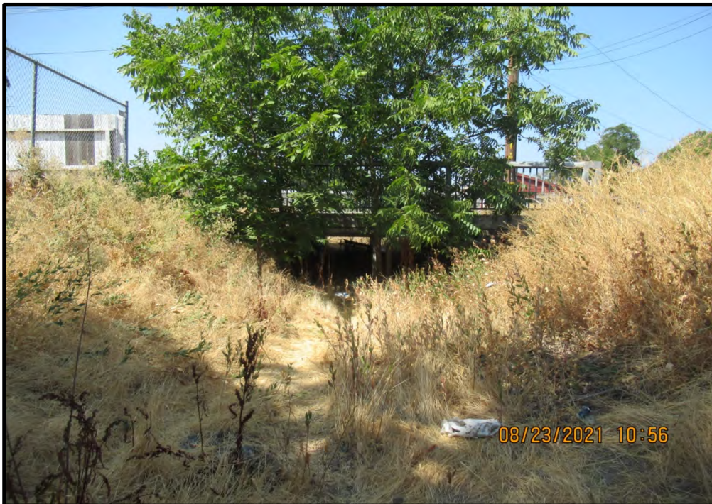
Bridge over Pock Lane, looking southwest from just north of the northwest corner of the site; 08/23/21. A new storm drain outfall may be constructed in Bieghle Drain.
