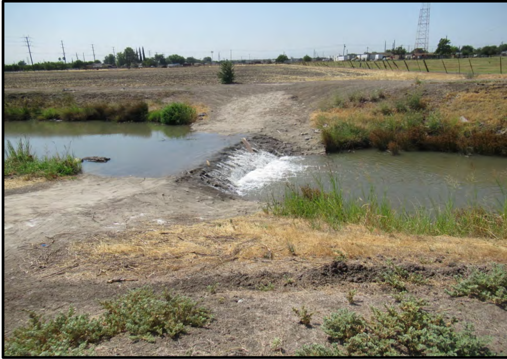
Low-flow crossing across Duck Creek, looking southeast from the south-central part of the site; 07/30/21.
