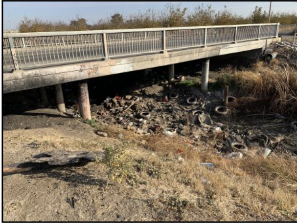
13 : View looking southeast showing bridge over dry canal adjacent to the property to the south.
