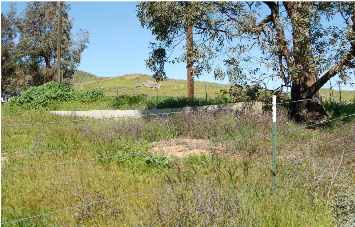
View of an old block retaining wall along the east side of the site
