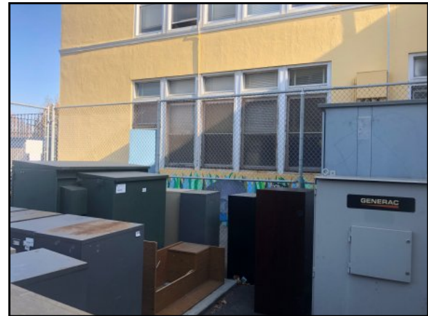
24 : View of the on-site transformers.
