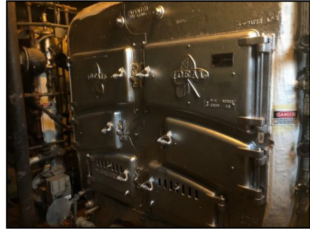
26 : View of a boiler in the boiler room.
