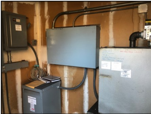
35 : View of the elevator equipment room.
