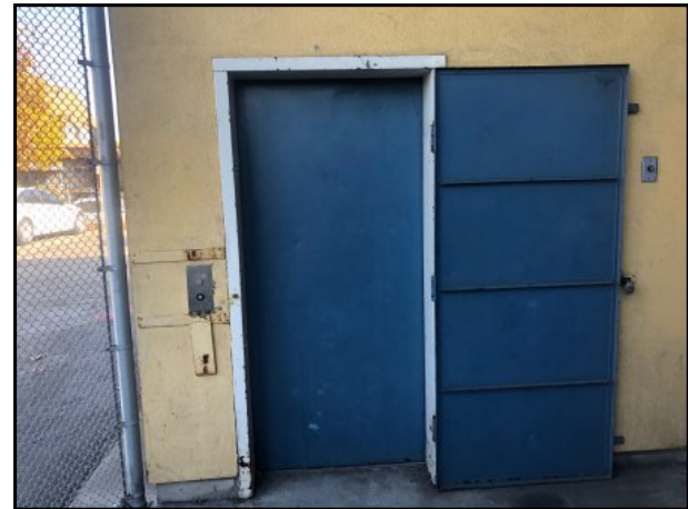
20 : View of the on-site elevator.
