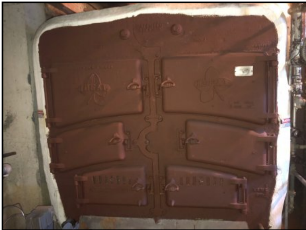
27 : View of a boiler in the boiler room.
