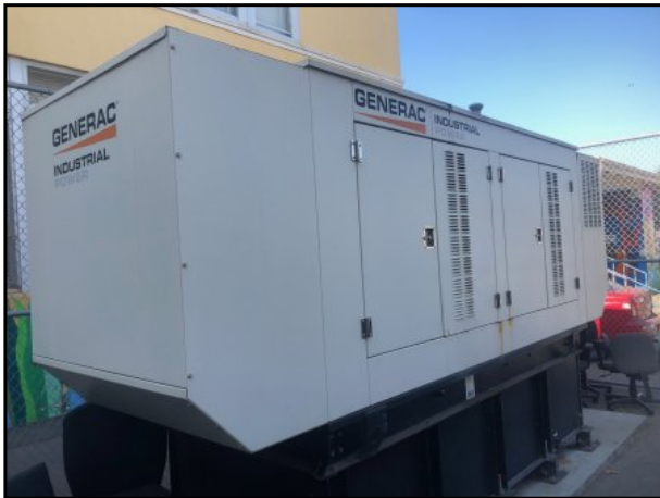
23 : View of the on-site generator.
