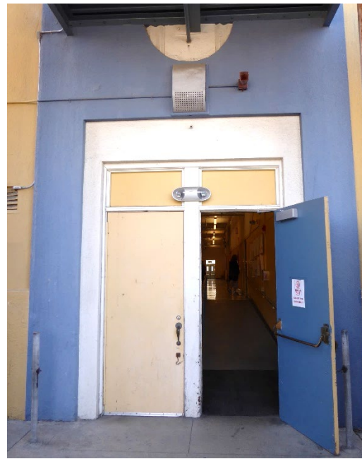
Figure 22: Looking south at entrance at rear of east wing. Note concrete detail where staircase is attached to façade.
