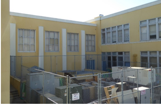
Figure 42: Fenced equipment storage area to immediate north of rear façade, looking southwest.
