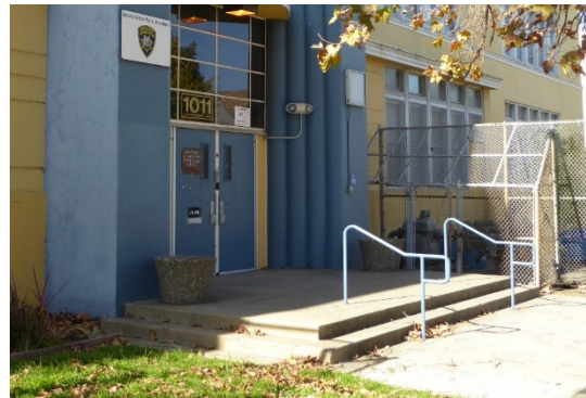
Figure 39: Concrete steps and landing with metal railings at main entrance, looking northwest.
