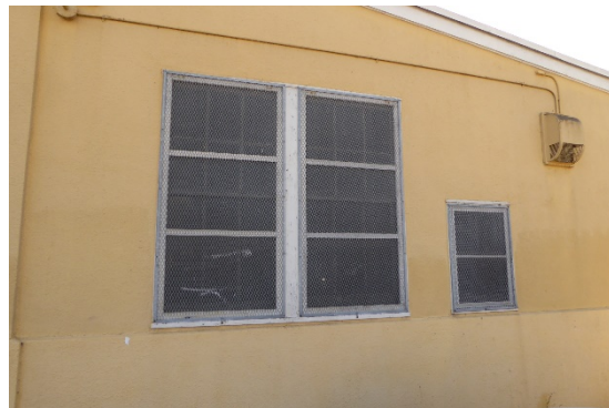
Figure 33: Paired and a smaller single wood-sash window at the west side of the north façade, looking south.
