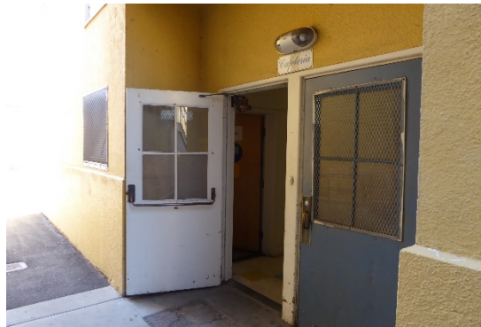
Figure 36: Looking northwest at recessed entrance at south façade featuring two flush- wood doors with four divided lites each.
