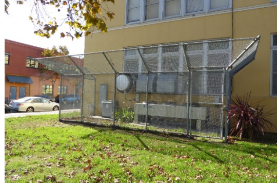
Figure 38: HVAC equipment enclosure at south end of primary façade, looking west.
