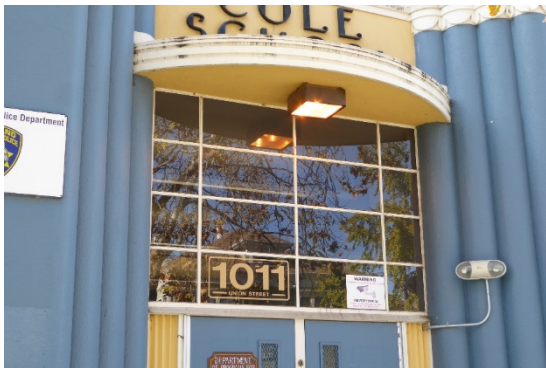
Figure 10: Divided-lite steel-frame window above main entrance, and curved entrance canopy, looking west.
