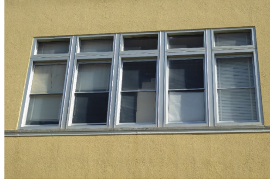
Figure 4: Typical second story windows without security screens.
