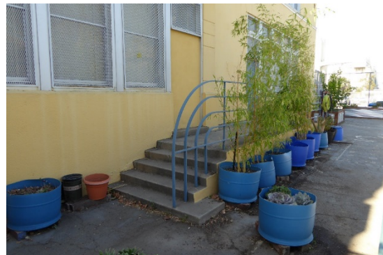
Figure 15: Concrete steps and landing with metal railing at the north end of the primary façade, looking northwest.
