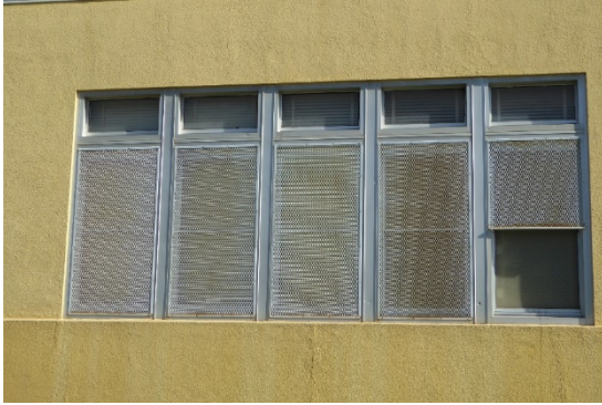
Figure 3: Typical first story windows with security screens.
