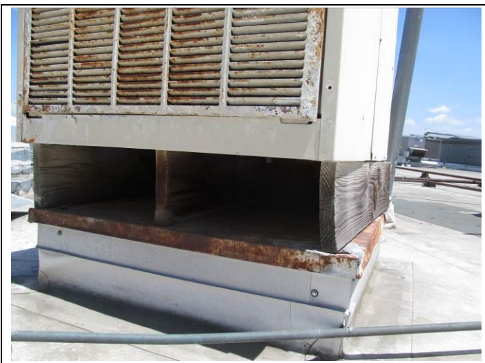
27. Equipment anchorage lacking
