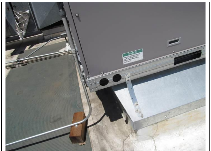
28. Acceptable equipment anchorage straps
