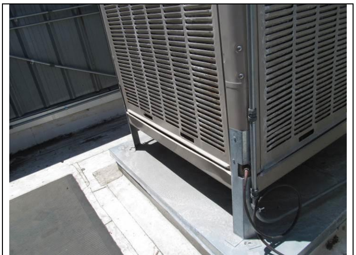
30. Equipment anchorage with sheet metal
