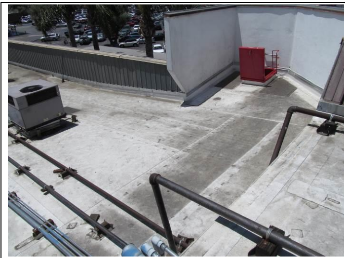
21. Continuously unbraced gas feed lines
