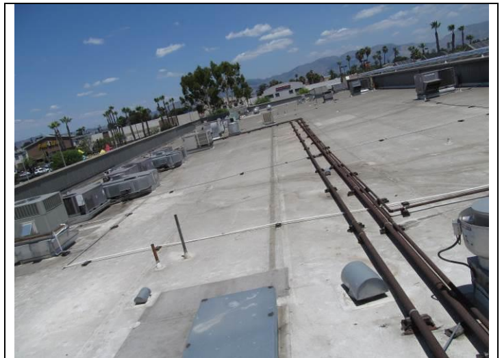
22. Continuously unbraced gas feed lines
