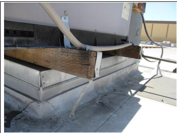
23. Equipment anchorage varies in quality
