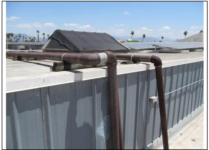
20. Continuously unbraced gas feed lines
