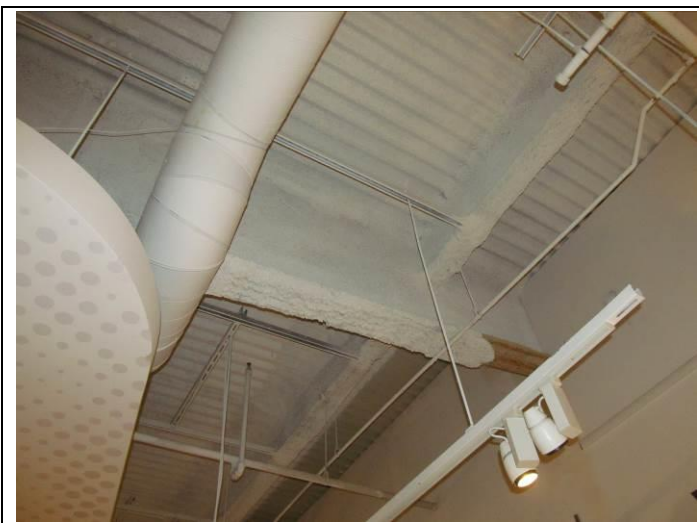
33. Exposed steel beam with fire safing scraped off of underside of flange
