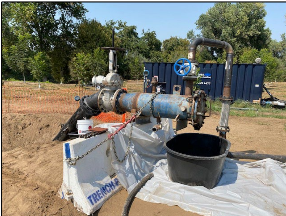
Figure 2-16. Photograph of a Sample Pig Receiver and Associated Equipment
