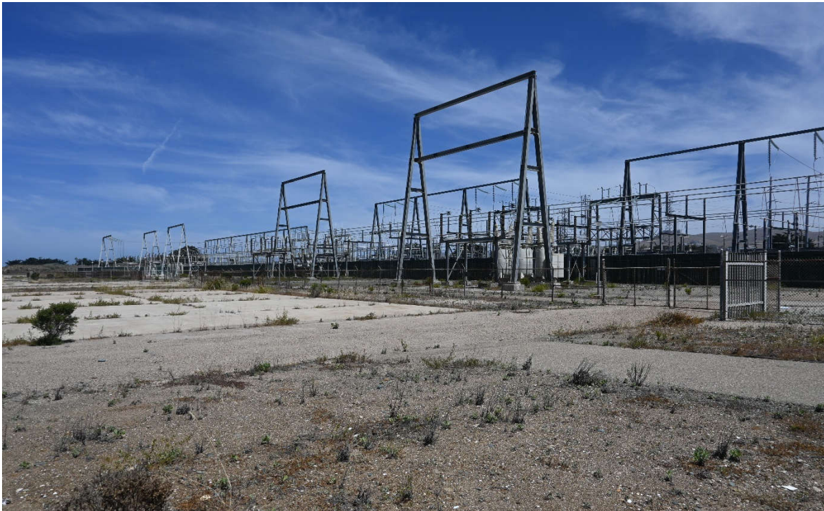
Figure 21 Overview of Switchyard, Facing Northwest
