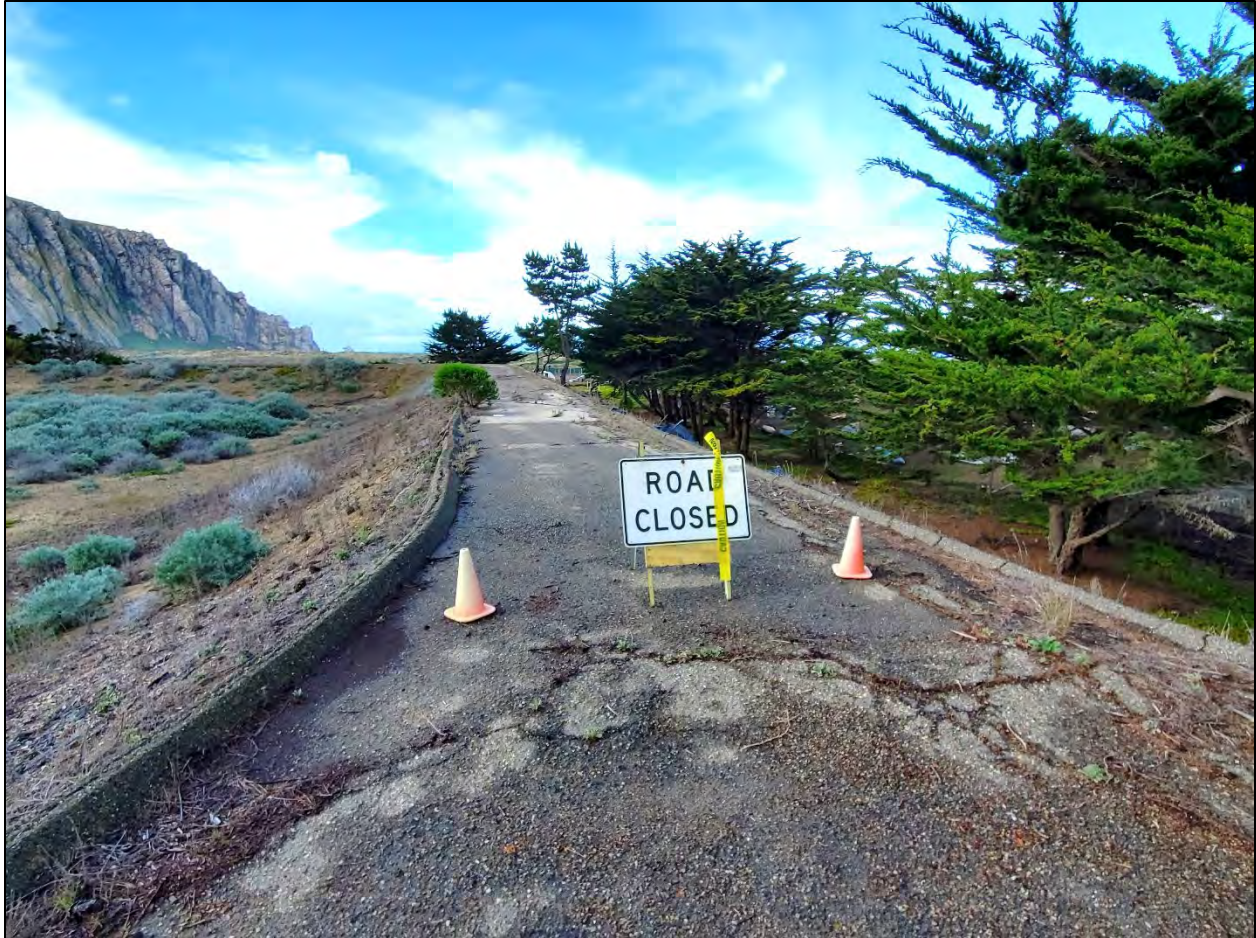
Photo 8: Image viewing west of one of the numerous asphalt paved roads atop an earthen berm within the Survey Area. March 11, 2021
