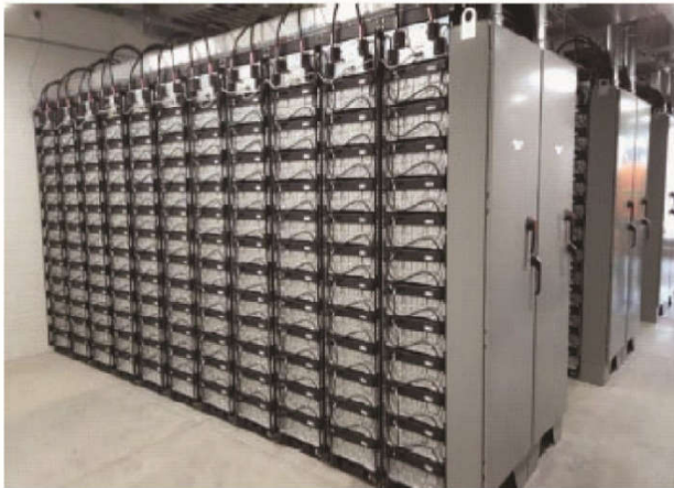
Battery Energy Storage
