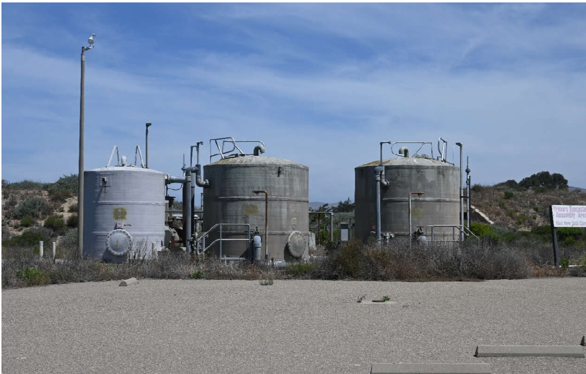
Figure 17 Sump Water Tanks, Facing West
