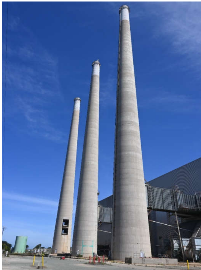
Figure 11 Boiler Stacks, Facing West from East Side of Generating Plant
