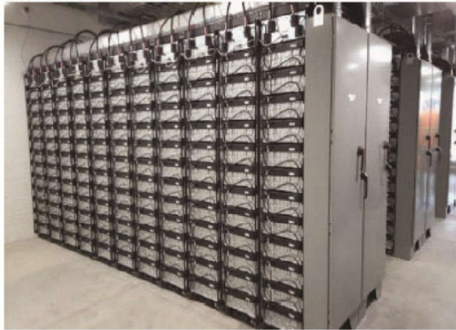
Battery Energy Storage
