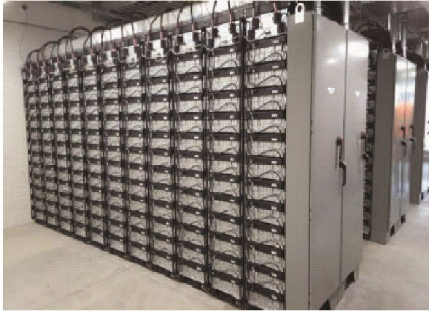
Battery Energy Storage
