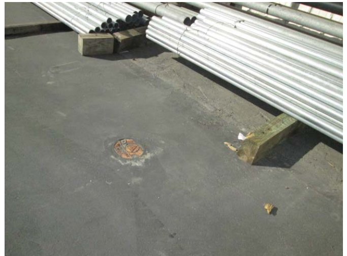
Picture 23 – Methane monitoring well on the east side of building #3
