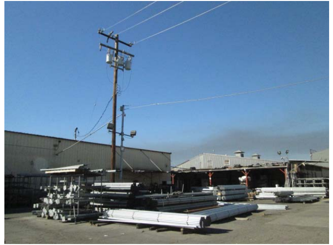
Picture 22 – Pole-mounted transformers
