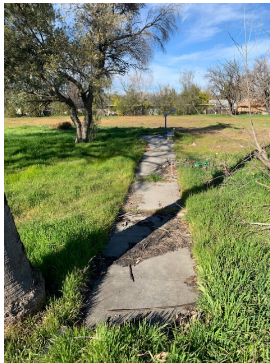
Sidewalk, view north
