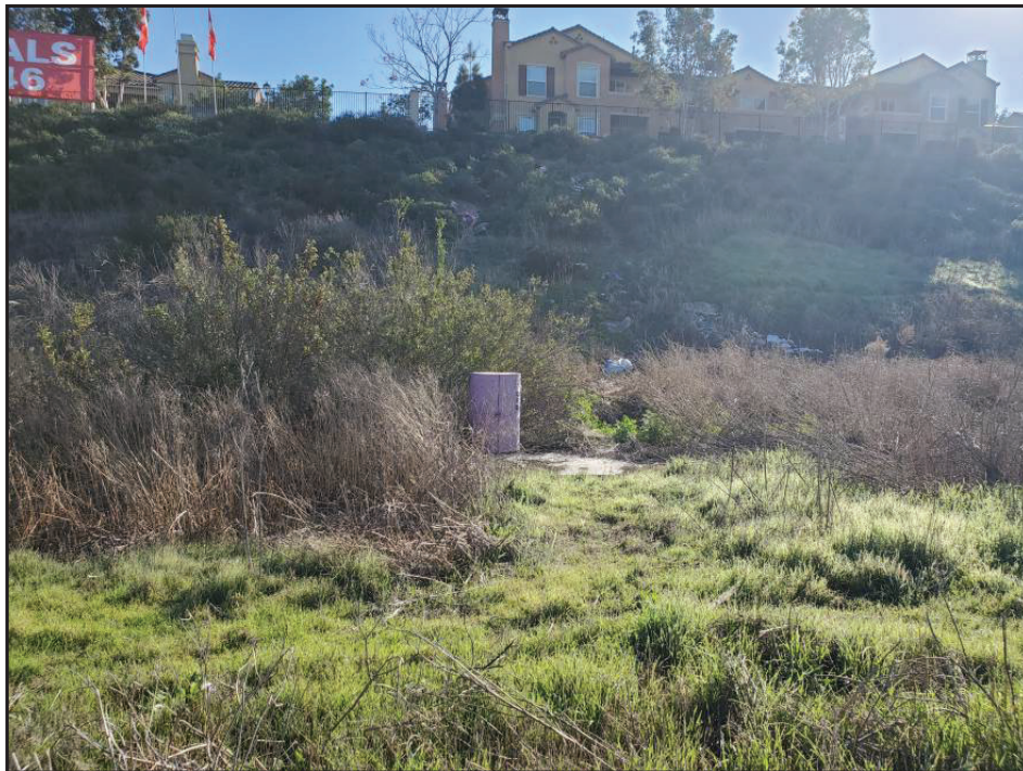
View of Otay Mesa Water District infrastructure along eastern boundary of the Subject Property.
