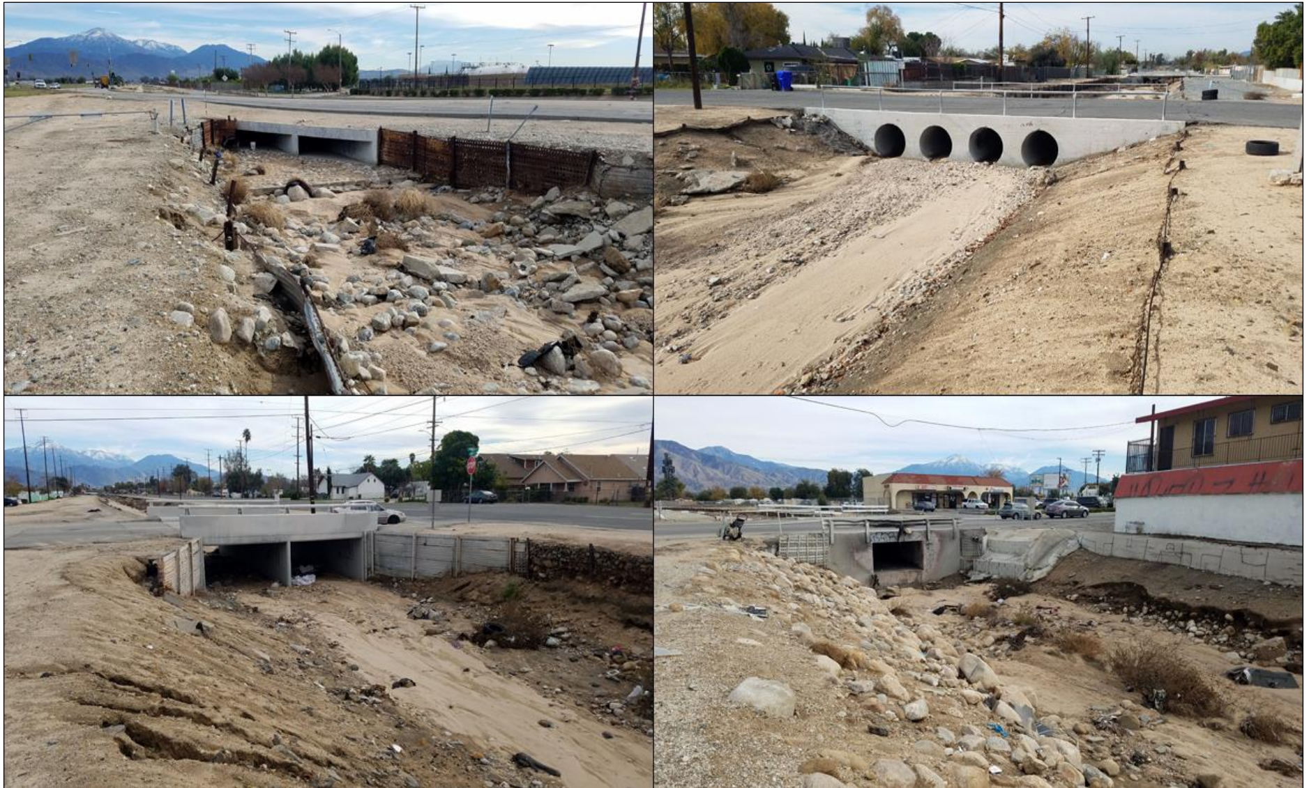
Typical bridges and culverts along the City Creek Channel. Clockwise from upper left: Third Street crossing, view to the east; Del Rosa Avenue crossing, view to the southwest; Tippecanoe Avenue crossing, view to the east; Pedley Road crossing, view to the southeast. (Photographs taken on December 10, 2019)
