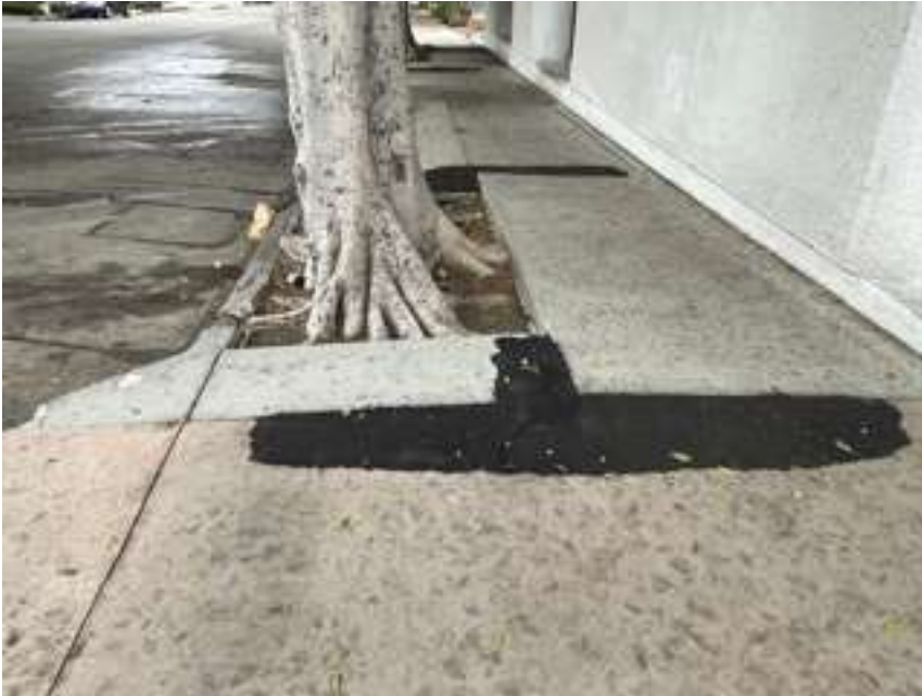
Tree number 3 with asphalt patches where it has grossly uplifted the adjacent sidewalk.
