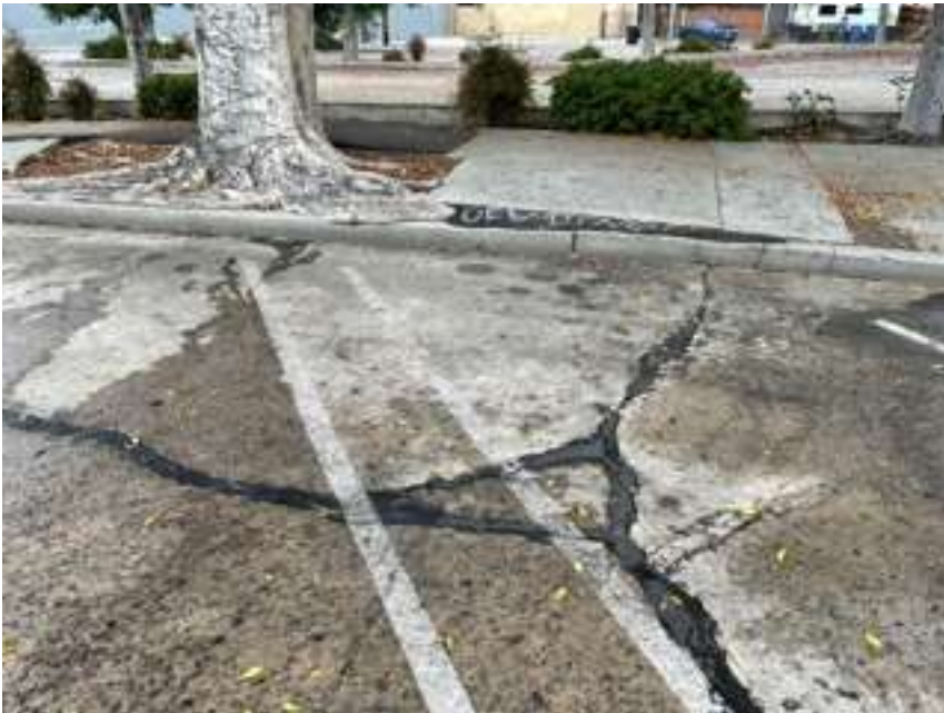
Tree number five uplifted adjacent street surface.
