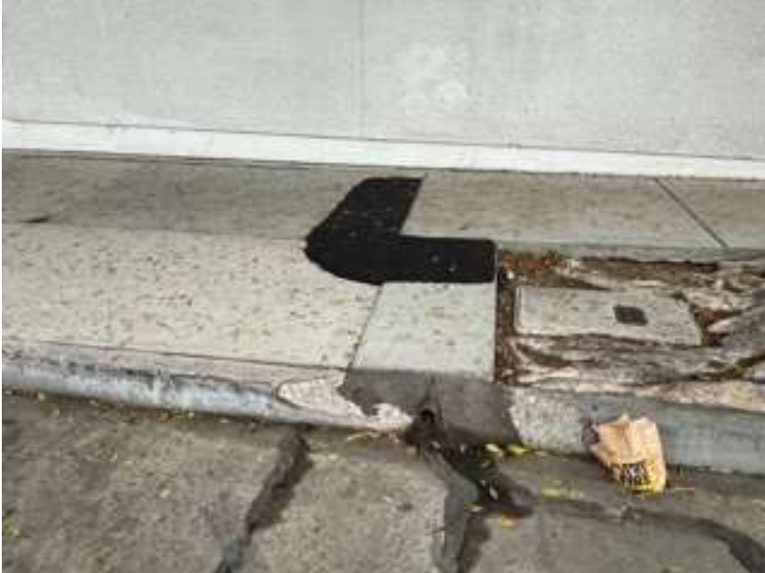
Tree number 3 at the eastern end of the planter frontage where it has been uplifted and patched.
