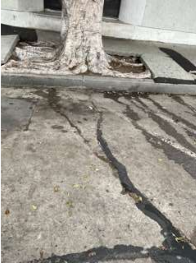
Fractured street surface adjacent to tree number four.
