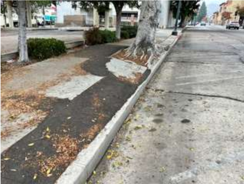
Tree number five where it has grossly uplifted the curb, sidewalk, and fractured adjacent street surface.
