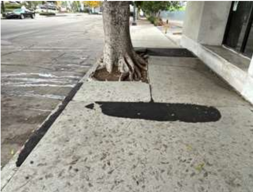
Tree number four where its surface rots have damaged adjacent sidewalk.
