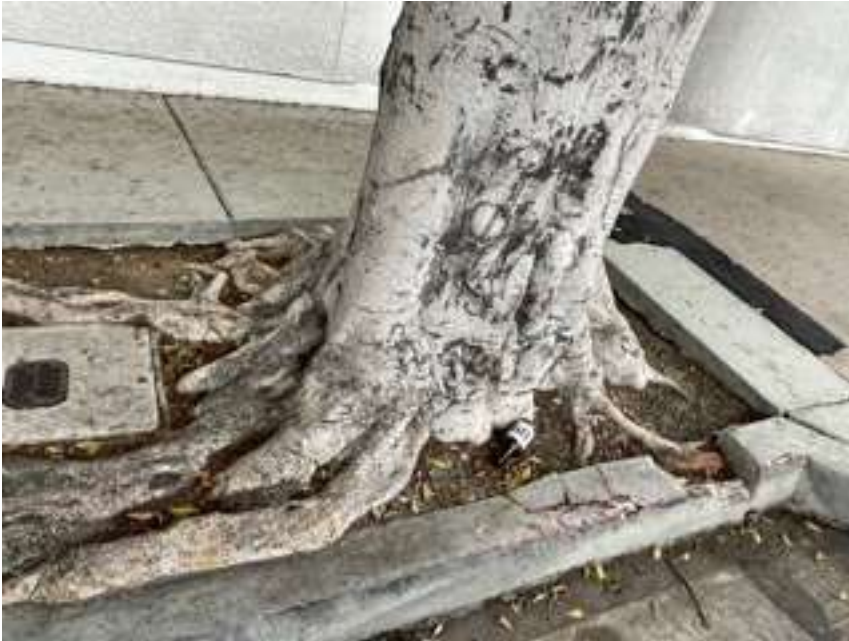
Tree number three where the curb along street frontage has been damaged by surface roots.
