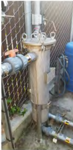
Intersil GWET Influent Bag Filtration Unit
