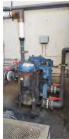
Siemens GWET Bag Filtration Units
