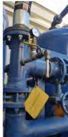
Siemens GWET Influent Sample Port
