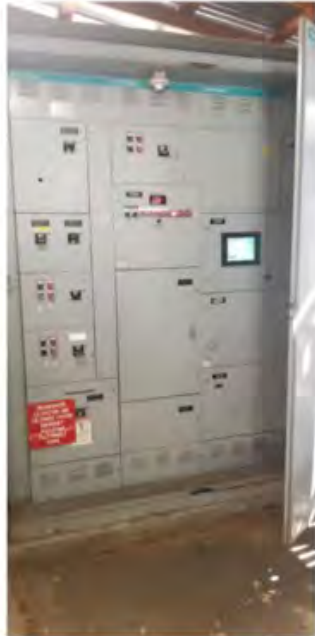
Siemens GWET System Control Panel
