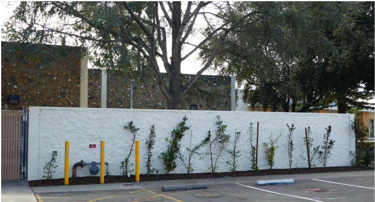
Figure 10. North façade of the west wing of the multipurpose building. Photograph taken 1/17/2022.
