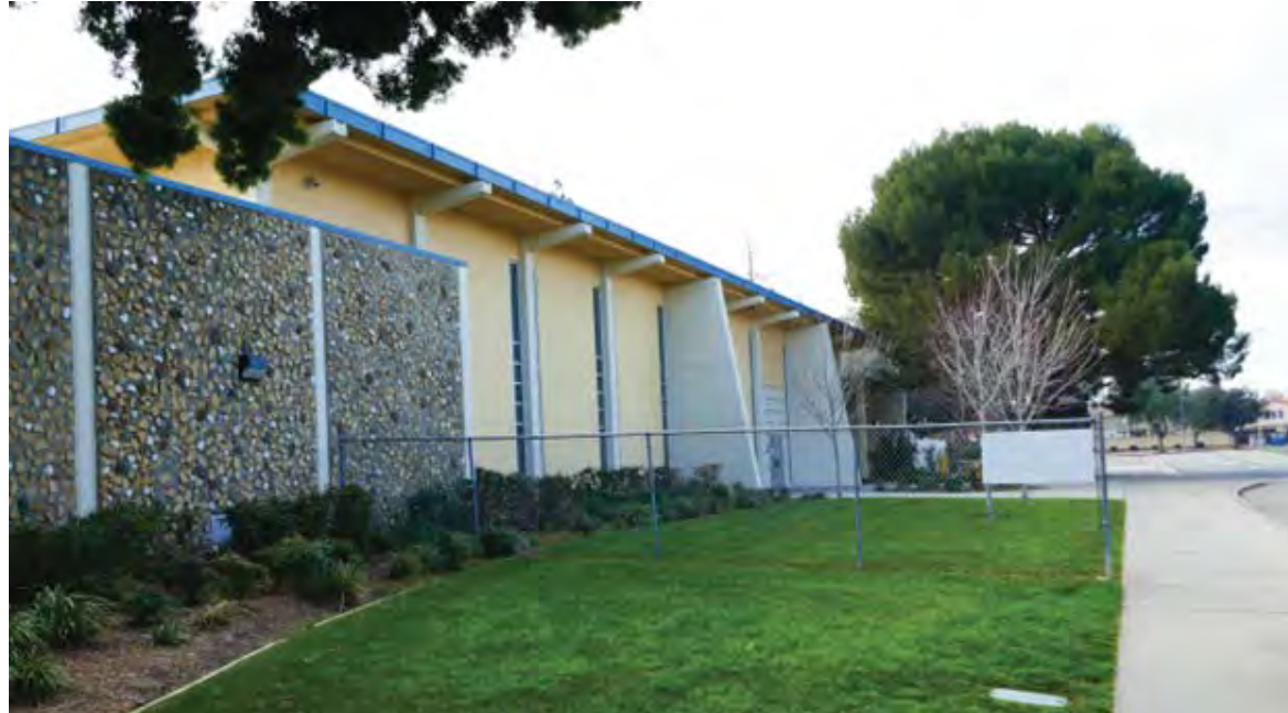
Photograph shows the scale of the buttresses and the exaggeration of the height of the building from the engaged columns buttresses. The façade of the east elevation can also be seen on the left. Camera facing west
