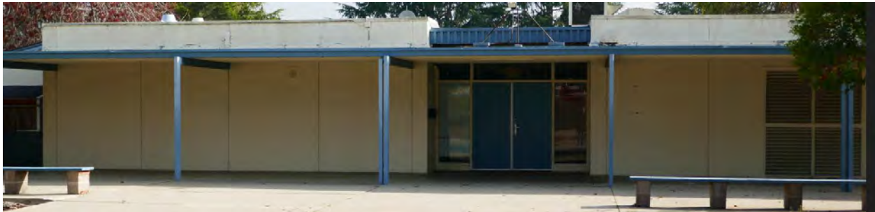
Figure 4. East elevation of building A on the west side of the central courtyard. Photograph shows typical plain wall type, typical recessed entry with roof detail, and the covered walkway design. Photograph taken 1/17/2022.
