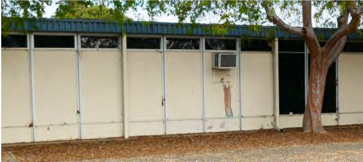
Figure 3. Detail of southern façade of building A, with typical metal-framed plywood and glass panels beneath the shallow eave and blue fascia. The two dark panels contain Aklo or plate glass. Photograph taken 1/17/2022.
