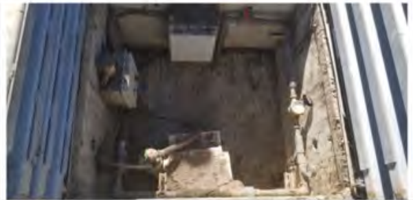
Intersil Extraction Well 12A Interior
