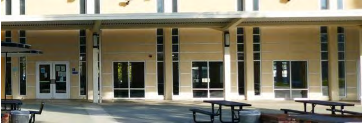
Figure 19. Detail of the multipurpose building fenestration and one of the doors, south elevation. Photograph taken 1/17/2022.
