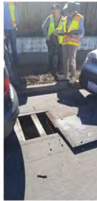
Siemens Extraction Well LR-1B (Off Site Study Area)
