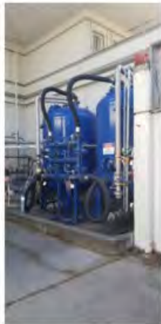
Siemens GWET GAC Vessels
