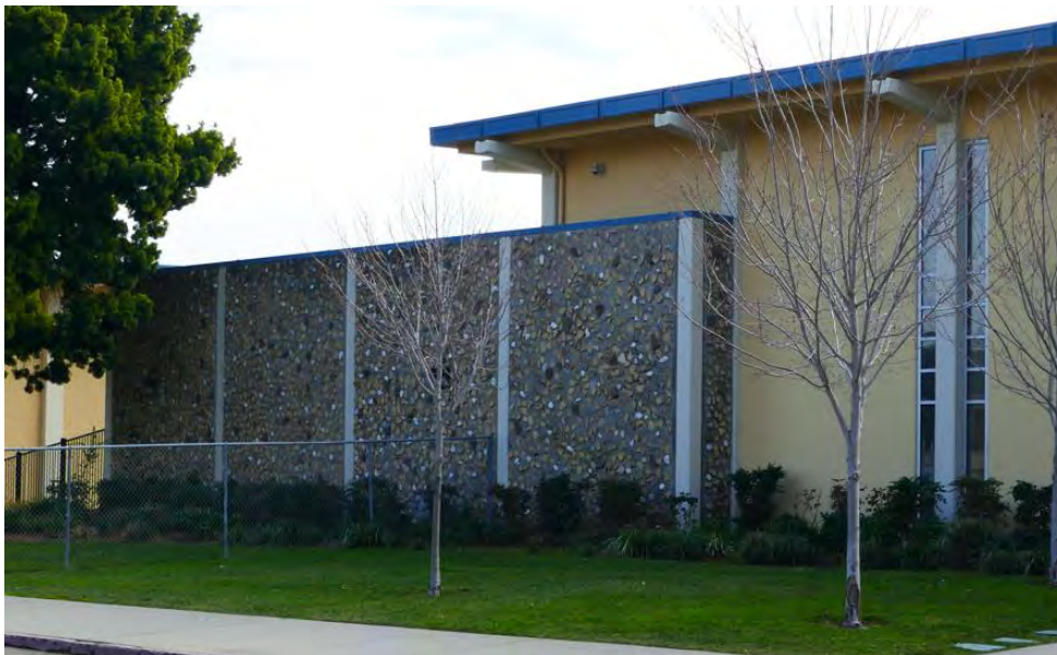
Figure 14. North façade of the east wing of the multipurpose building. Photograph taken 1/17/2022.
