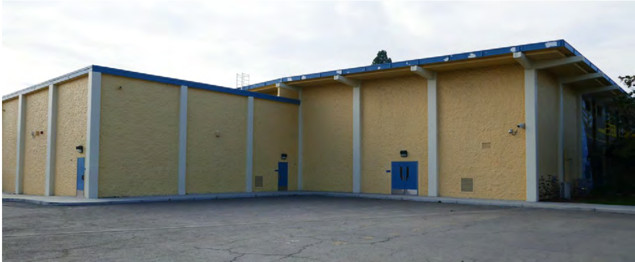
Figure 23. East elevation of the gymnasium with the addition. Camera facing southwest. Photograph taken 1/17/2022.
