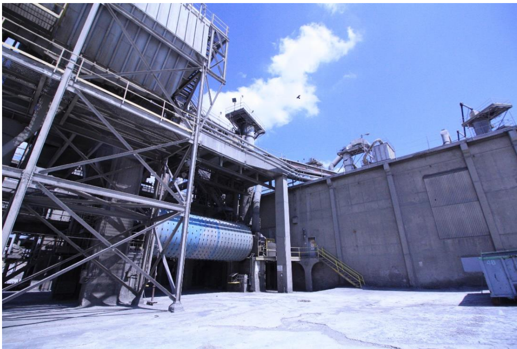
Figure 27: View of the ball grinding mill at the west elevation, view east.
