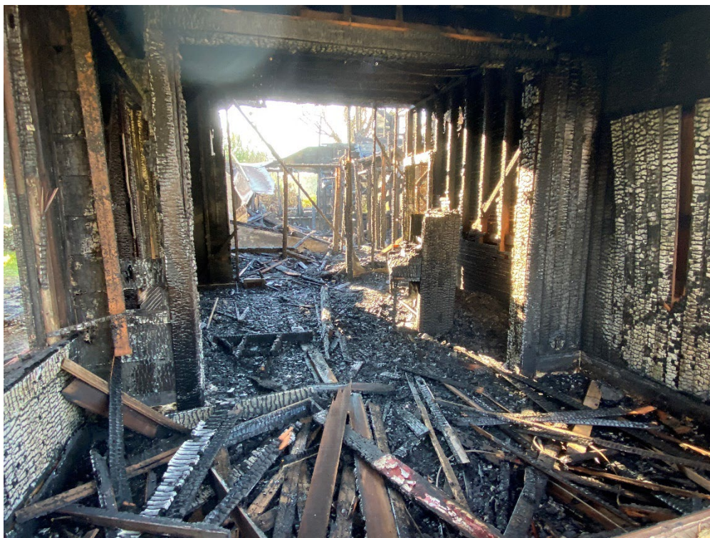
Photograph 18: Photograph of the burnt house in the central portion of the project site.
