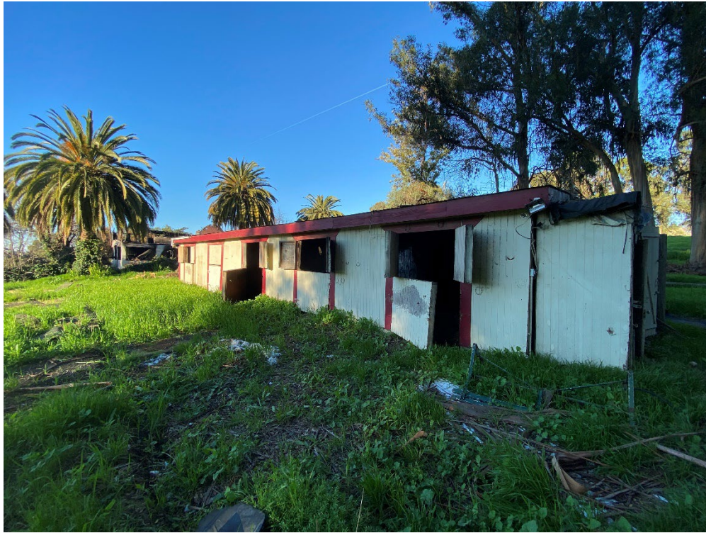
Photograph 37: A photograph of stables in the central portion of the project site.
