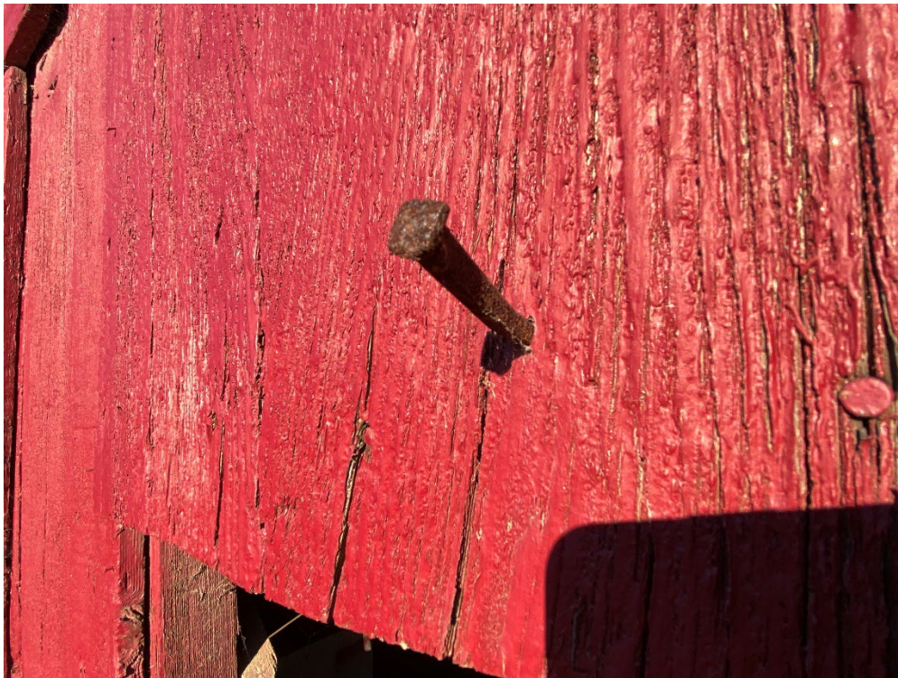
Photograph 32: An older nail that was added to the exterior of the red barn in the central portion of the project site. This nail was not part of the original construction of the barn
