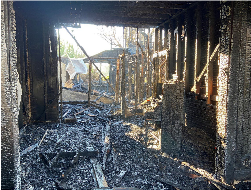
Photograph 19: Photograph of the burnt house in the central portion of the project site.
