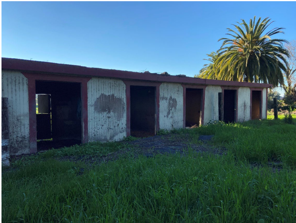
Photograph 34: A photograph of stables in the central portion of the project site.
