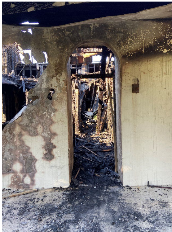
Photograph 22: An interior photograph of the burnt house located in the central portion of the project site.
