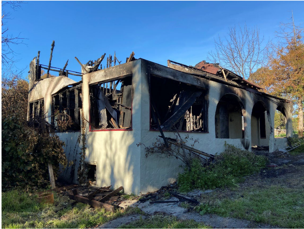
Photograph 21: A burnt house located in the central portion of the project site.
