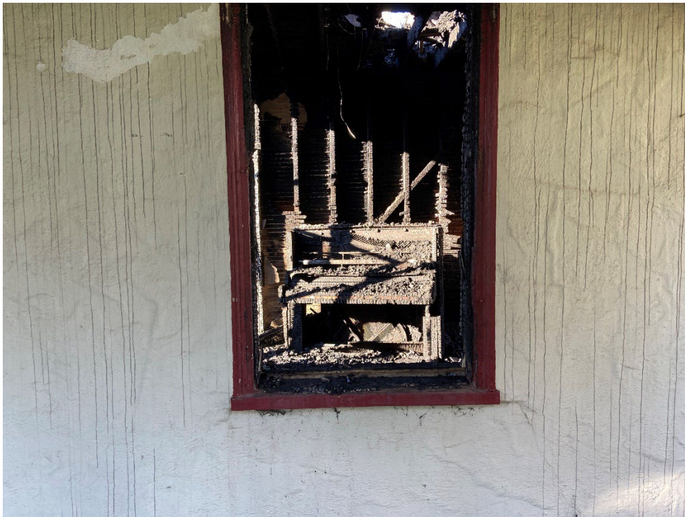
Photograph 24: An interior photograph of the burnt house located in the central portion of the project site
