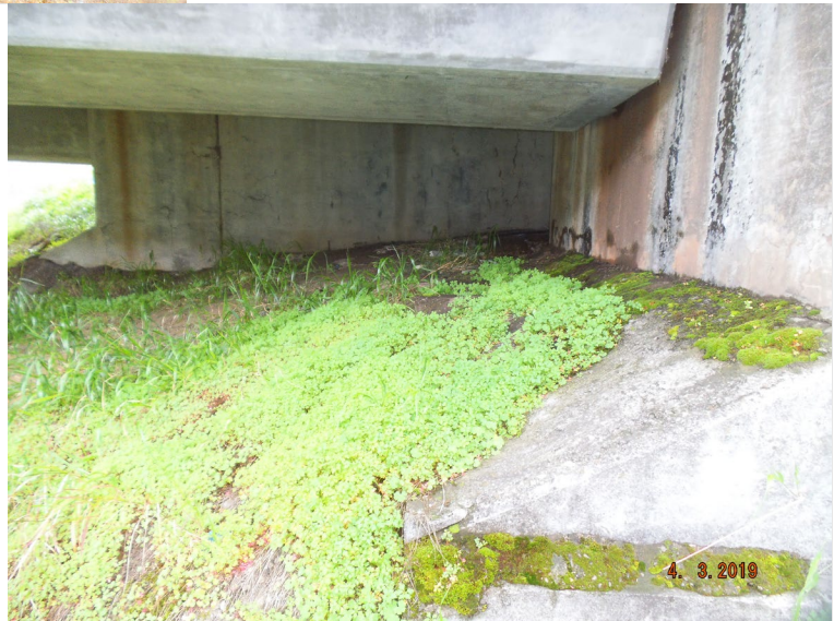
Figure 4. Views of Erosion and Drainage Problems at Concord Project Sites
