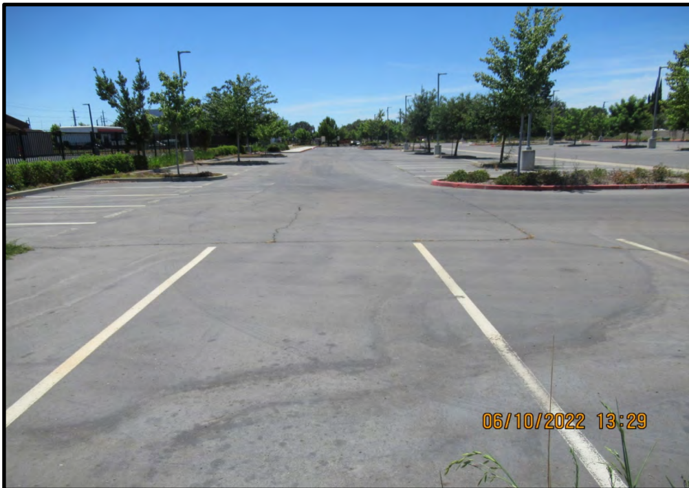
Existing parking lot where utilities relating to the new parking areas will be trenched underground, looking southwest from the southwest part of the East Parking Lot site; 06/10/22.
