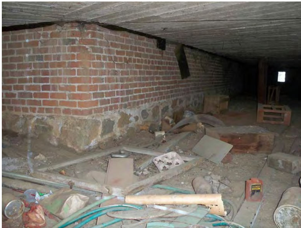
Casa Blanca Ranch house (Feature 1), crawl space under porch. View to southeast, 8/17/2012.
