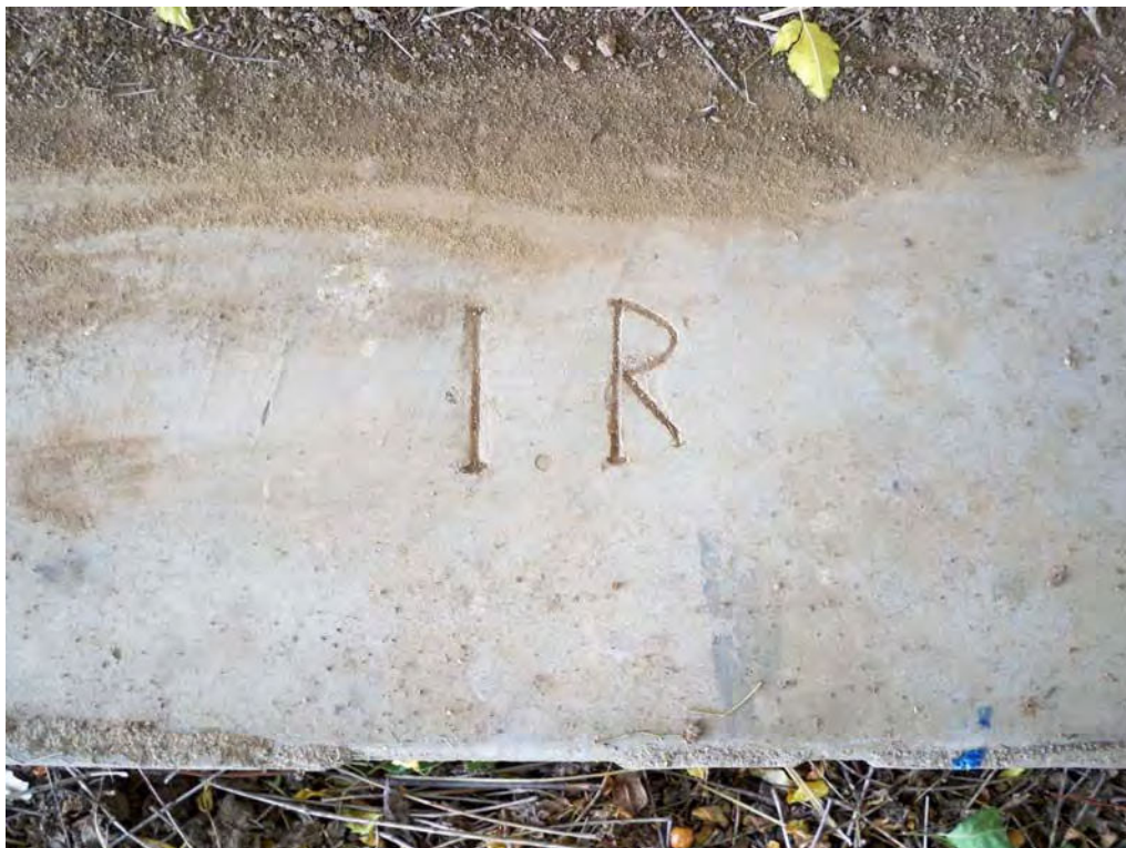
"IR" inscribed in original back porch of Rodriguez house (Feature 5). View to east, 8/17/2012.
