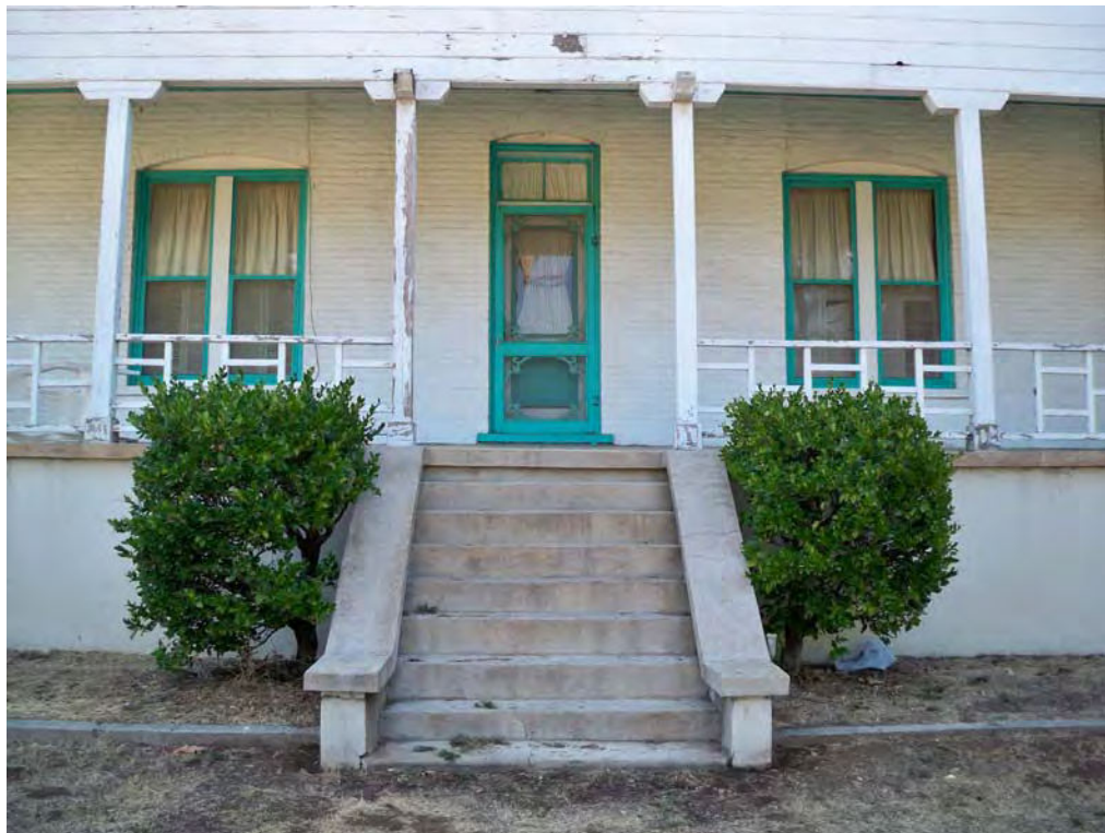
Casa Blanca Ranch house (Feature 1), main entry in west elevation. View to east, 8/17/2012.
