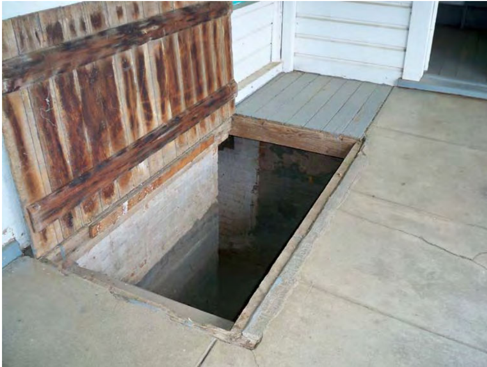
Casa Blanca Ranch house (Feature 1), trap door to rear basement in north side porch View to southwest, 8/17/2012.
