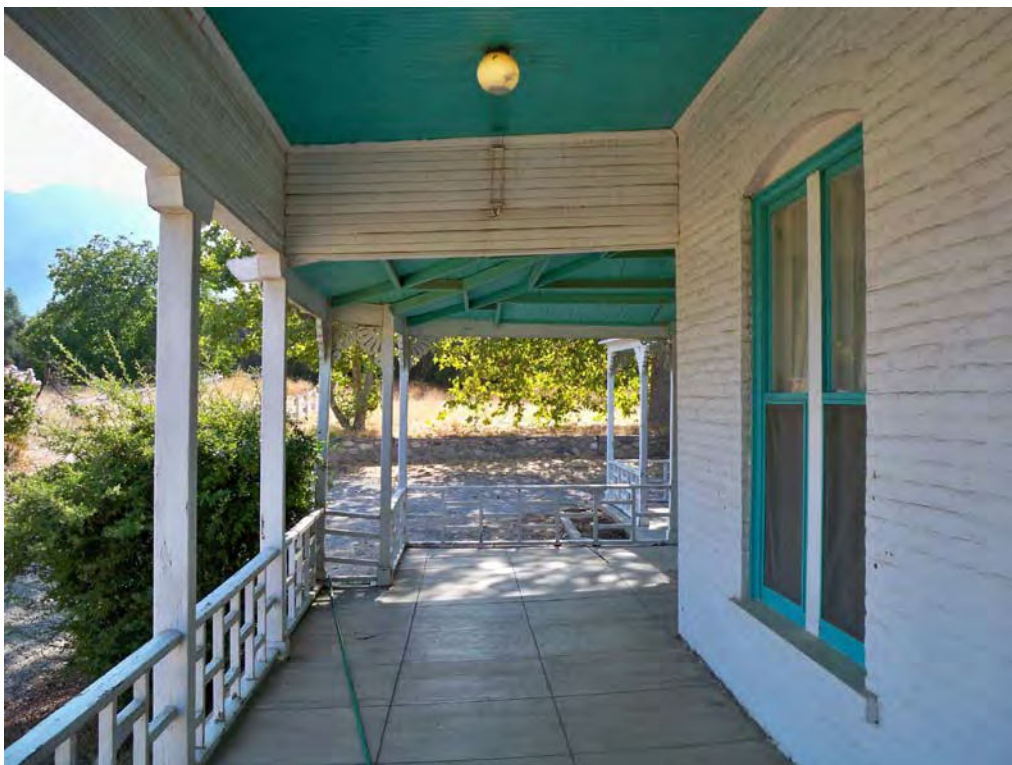
Casa Blanca Ranch house (Feature 1), porch along north side. View to east, 8/17/2012.
