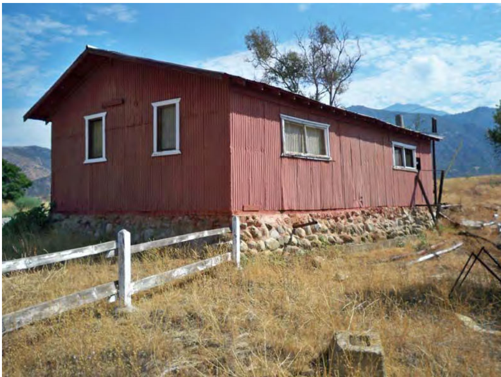
Blacksmith shop/service garage (Feature 4), west and rear (south) elevations. View to northeast, 8/17/2012.
