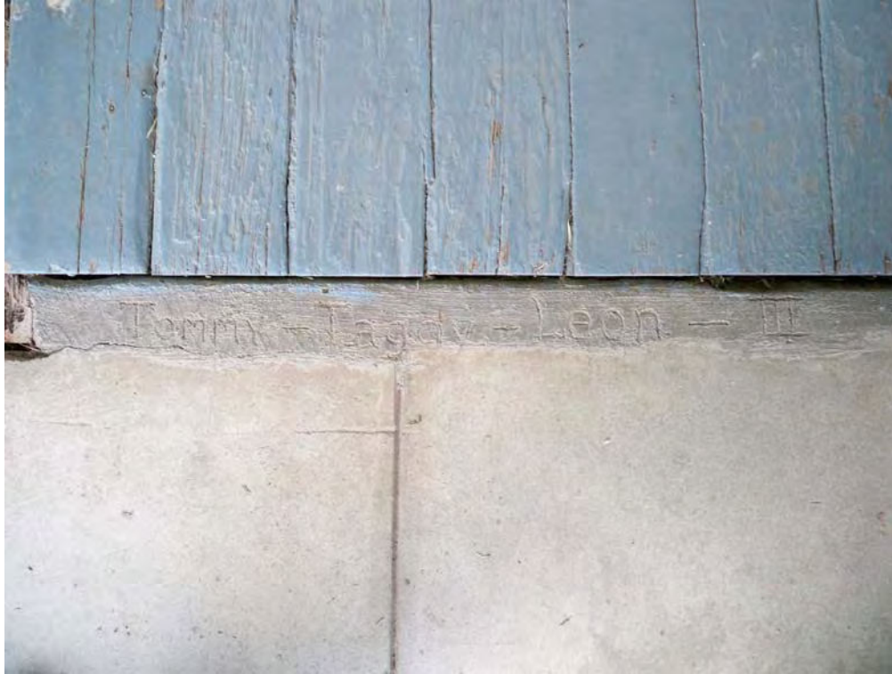
Casa Blanca Ranch house (Feature 1), "Tommy - Taggy - Leon - III" inscribed in concrete patch by trap door to rear basement in north side porch. View to south, 8/17/2012.
