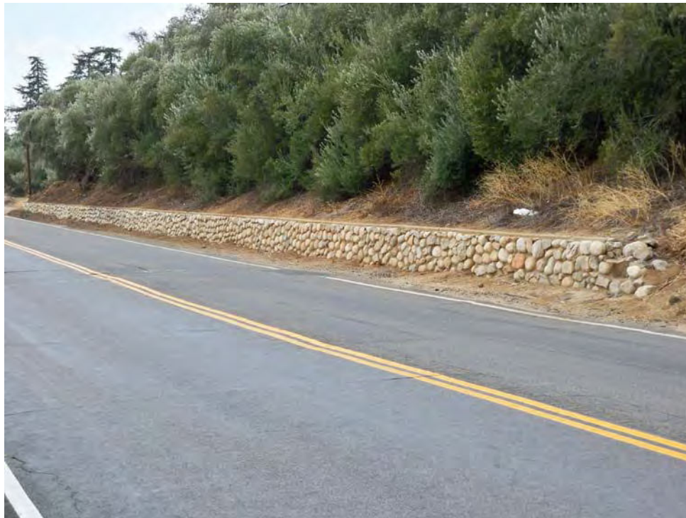
Stone retaining wall (Feature 13) on north side of Oak Glen Road. Olive grove (Feature 37) in background. View to northwest, 8/17/2012.
