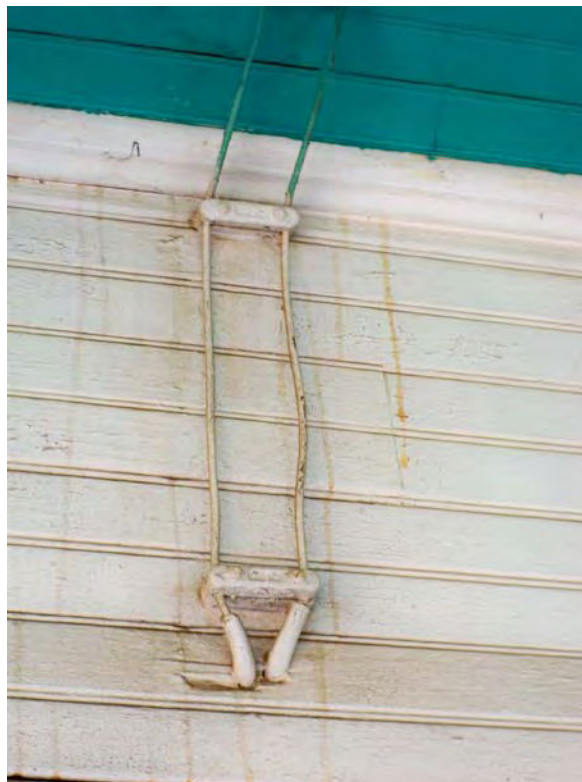
Casa Blanca Ranch house (Feature 1), original electrical wiring in north side porch. View to east, 8/17/2012.
