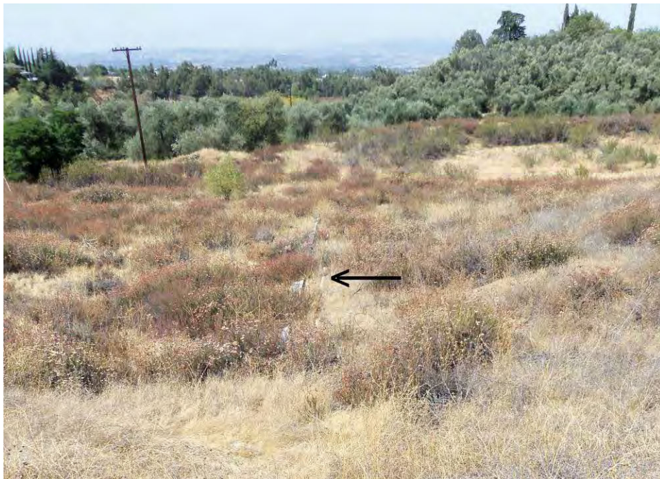
Concrete and rock flume (Feature 12e) between dam (Feature 12a) and holding pond (Feature 12f). View to southwest, 8/15/2012.
