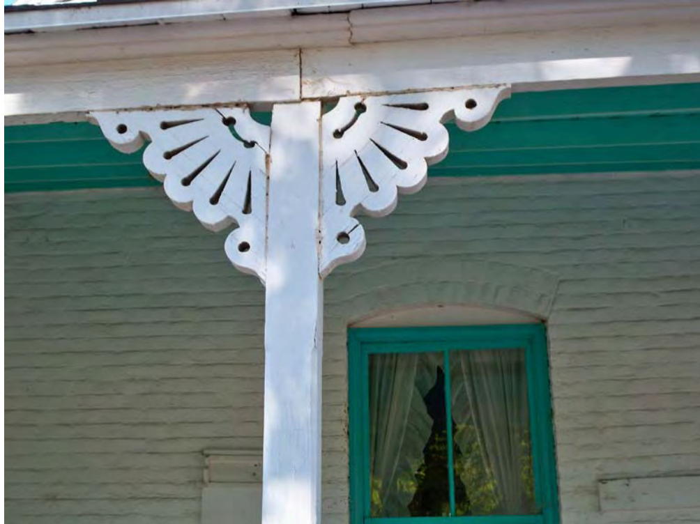
Casa Blanca Ranch house (Feature 1), porch brackets on north side View to south, 8/17/2012.
