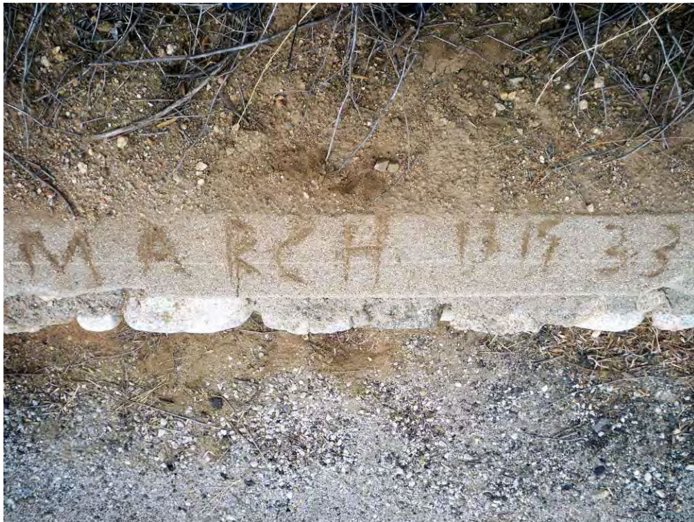
"March 13 1933" inscribed in top of stone retaining wall (Feature 13). View to north, 8/17/2012.
