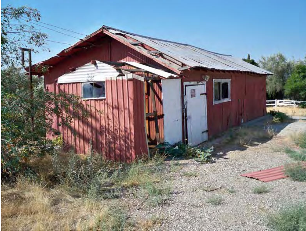
Blacksmith shop/service garage (Feature 4), east and north (front) elevations. View to southwest, 8/17/2012.
