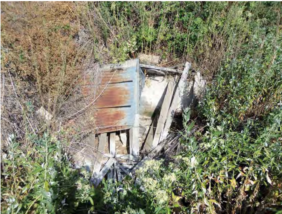
Concrete weir box with collapsed roof (Feature 22e), east of concrete reservoir (Feature 22d). View to northeast, 8/15/2012.
