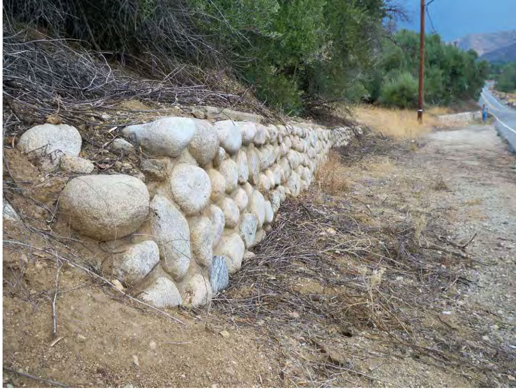
Stone retaining wall (Feature 13) on north side of Oak Glen Road. View to east, 8/17/2012.
