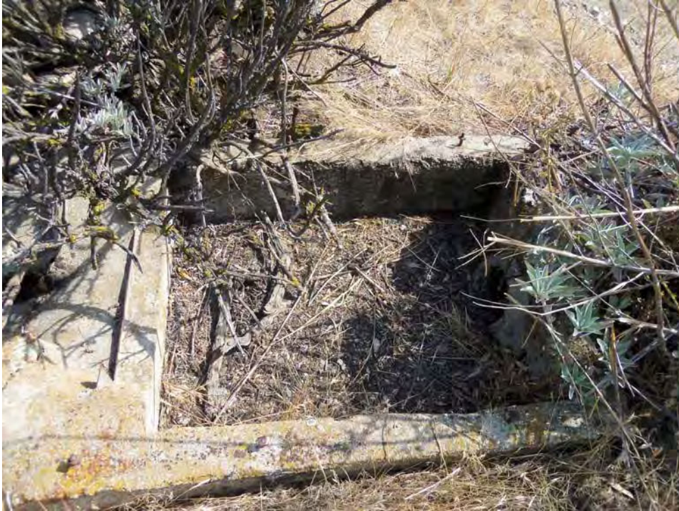
Concrete weir box attached to concrete reservoir (Feature 22d). View to south, 8/15/2012.
