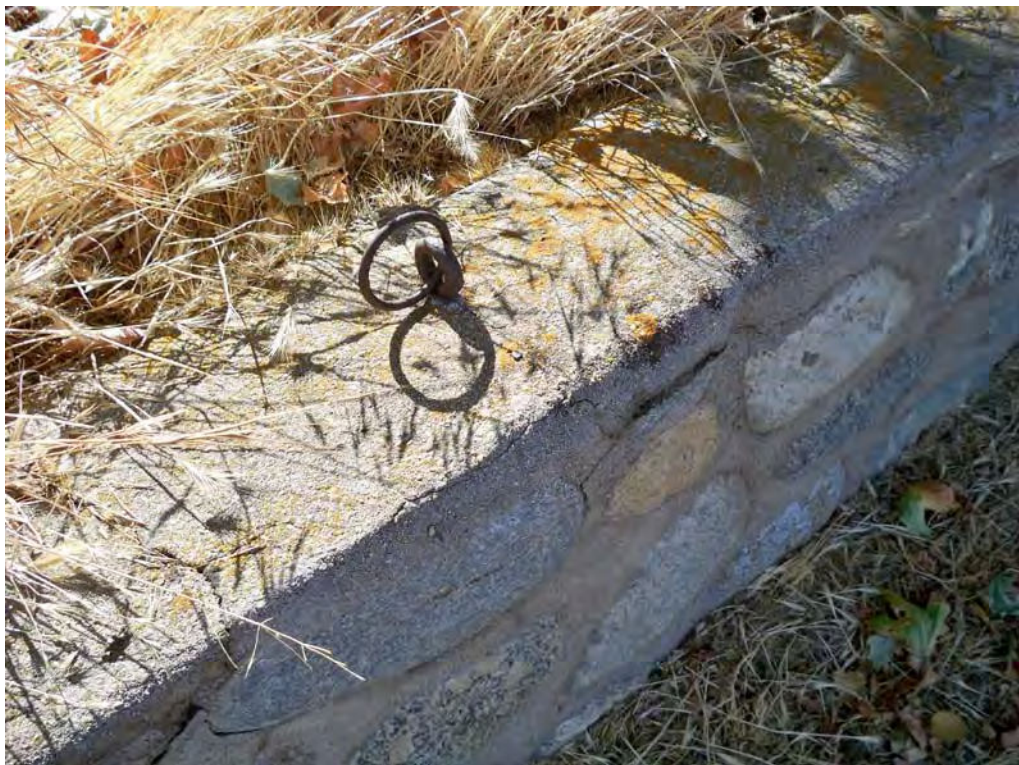
One of four rings for tethering horses in stone retaining wall (Feature 8). View to southeast, 8/17/2012.
