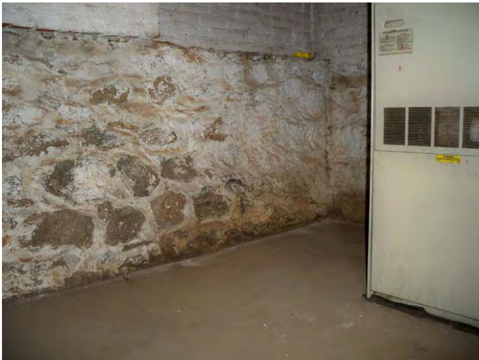
Casa Blanca Ranch house (Feature 1), Stone footing and brick walls inside rear basement. View to southwest, 8/17/2012.
