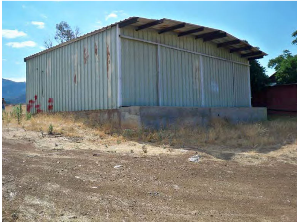
Modern prefabricated metal building (Feature 6), north and west elevations. View to southeast, 8/17/2012.
