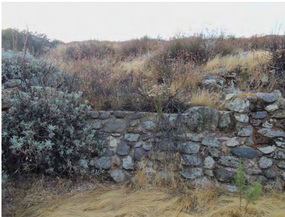
Stone retaining wall in ravine in northwest quarter of site (Feature 24). View to southeast, 8/16/2012.
