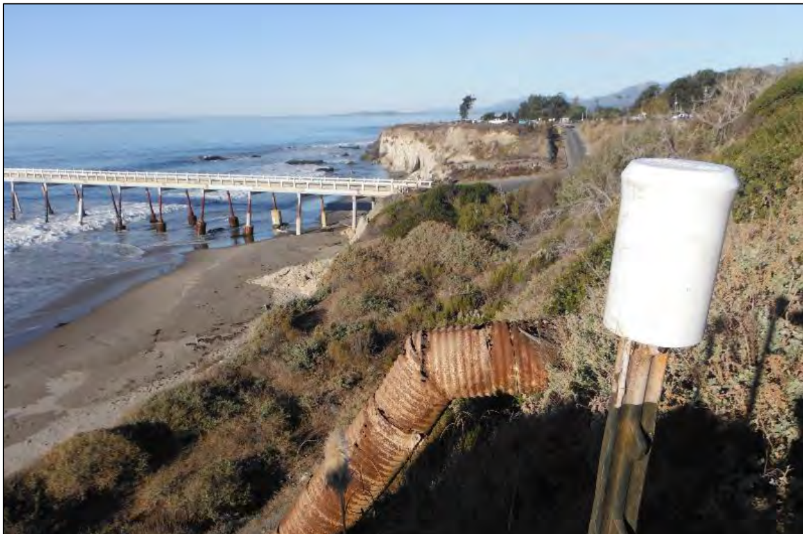
Photo 2. East side of Casitas Pier with Gail and Grace pipeline bundle (buried) and exposed concrete armament. Date: April 20, 2021, aspect west.
