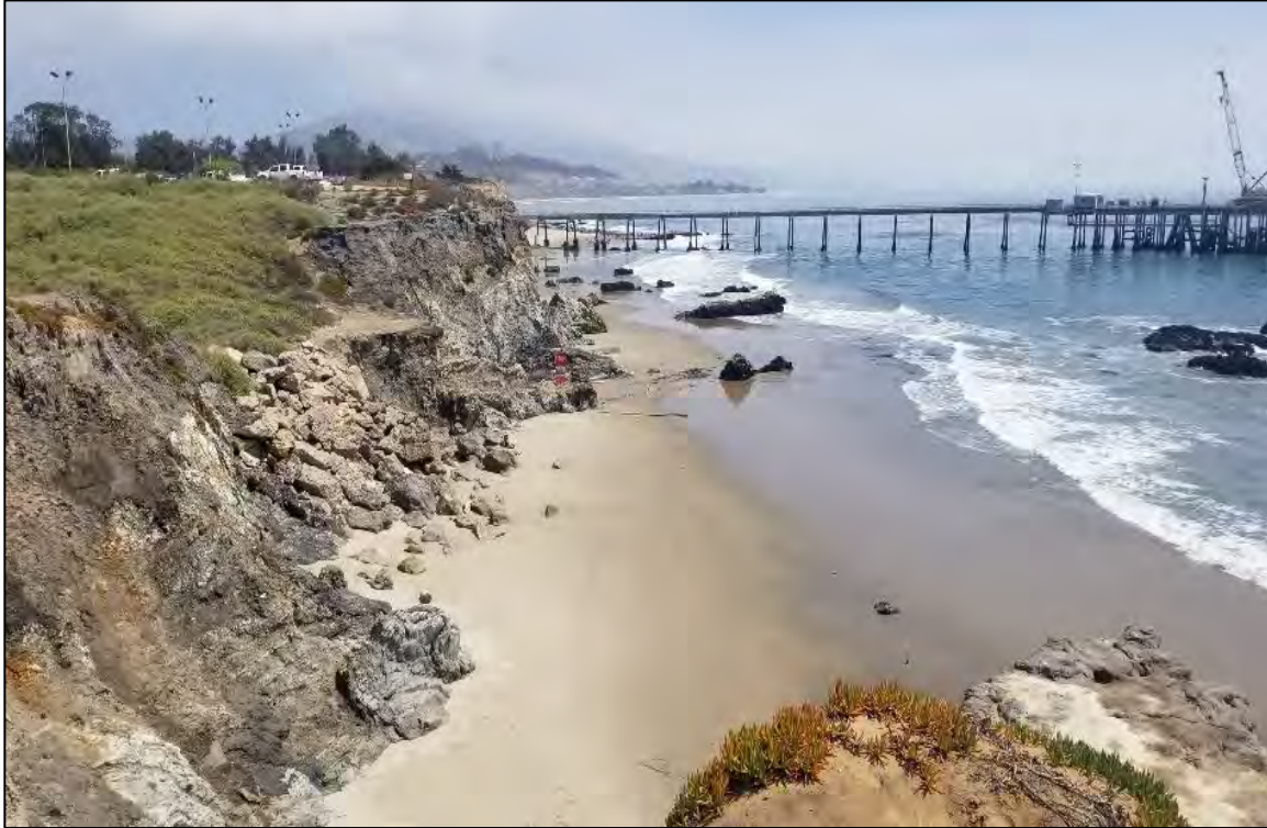
Photo 1. West side of Casitas Pier and Marketing and Marine Terminal pipeline bundle area (buried). Date: April 20, 2021, aspect east.
