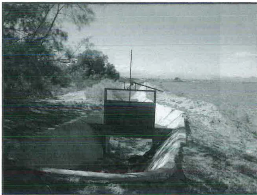
At the origin of the east-west portion of WSM Pump 6, looking west at the metal check
