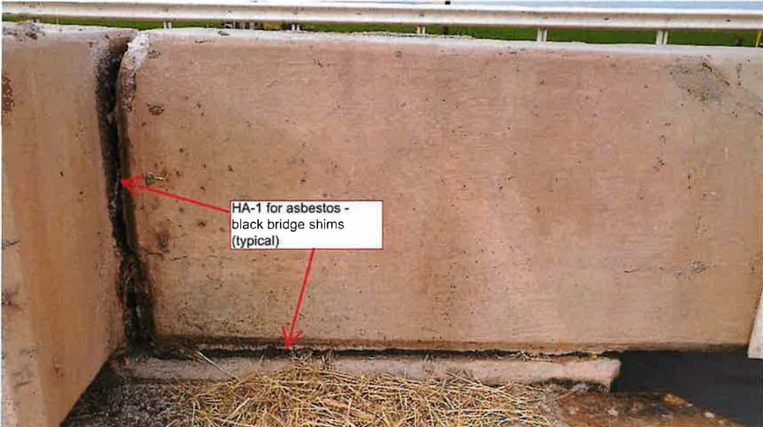
Photograph 17: Location of potential-asbestos containing material.
