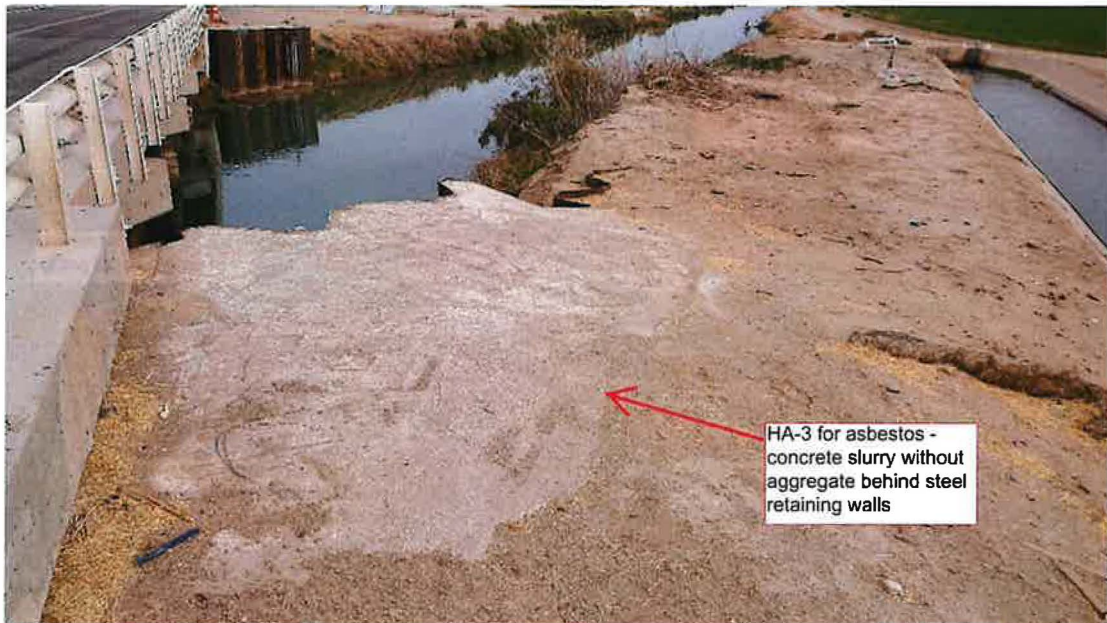
Photograph 13: Location of potential asbestos-containing material adjoining the bridge.
