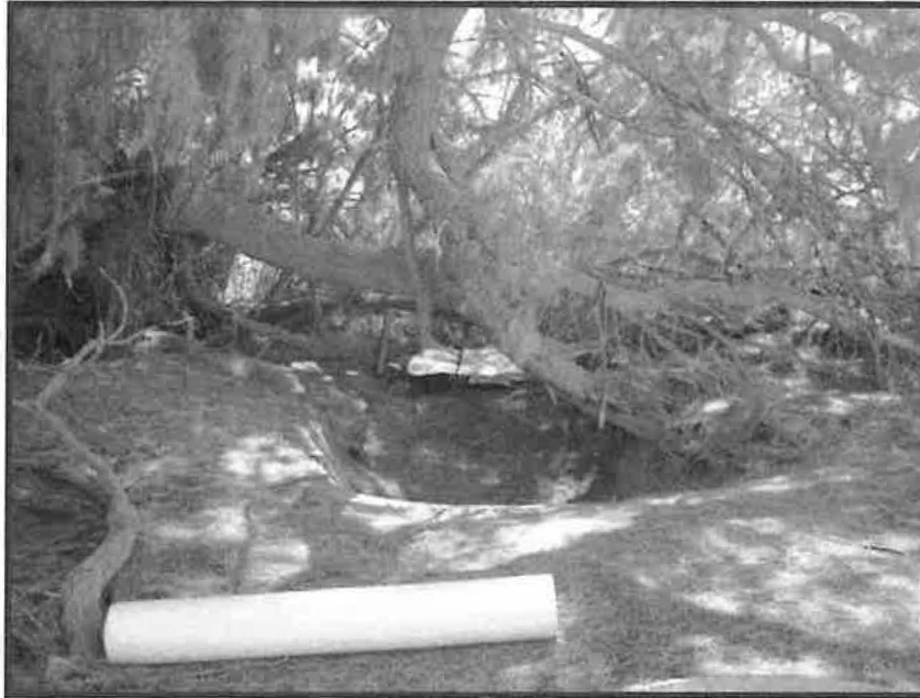
At the origin of the east-west portion looking south at concrete-lined structure
