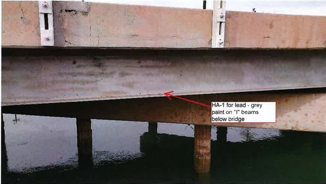
Photograph 16: Location of potential lead-containing paint.
