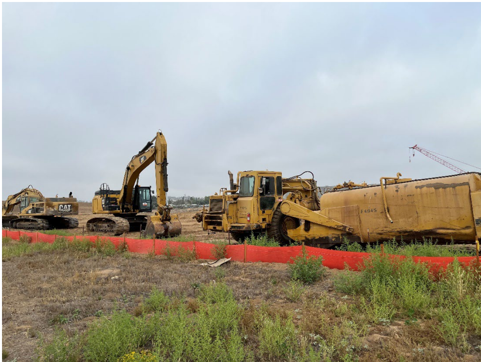
Photo 4 – Heavy equipment on adjoining site to the west, where grading activities were ongoing.
