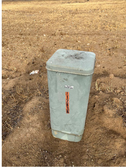
Photo 13 – Telecommunication box along eastern side of Property.
