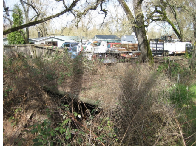
Photo 8: Unused steel and concrete bridge over Roseland Creek. The vehicles parked in the background are on the adjacent property.
