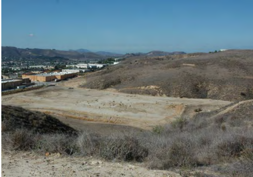
Photo 6 – Looking Southwest Across the Western Building Pad. Note hillside to the west is downhill and generally these fuels are light in part due to past wildfire activity.
