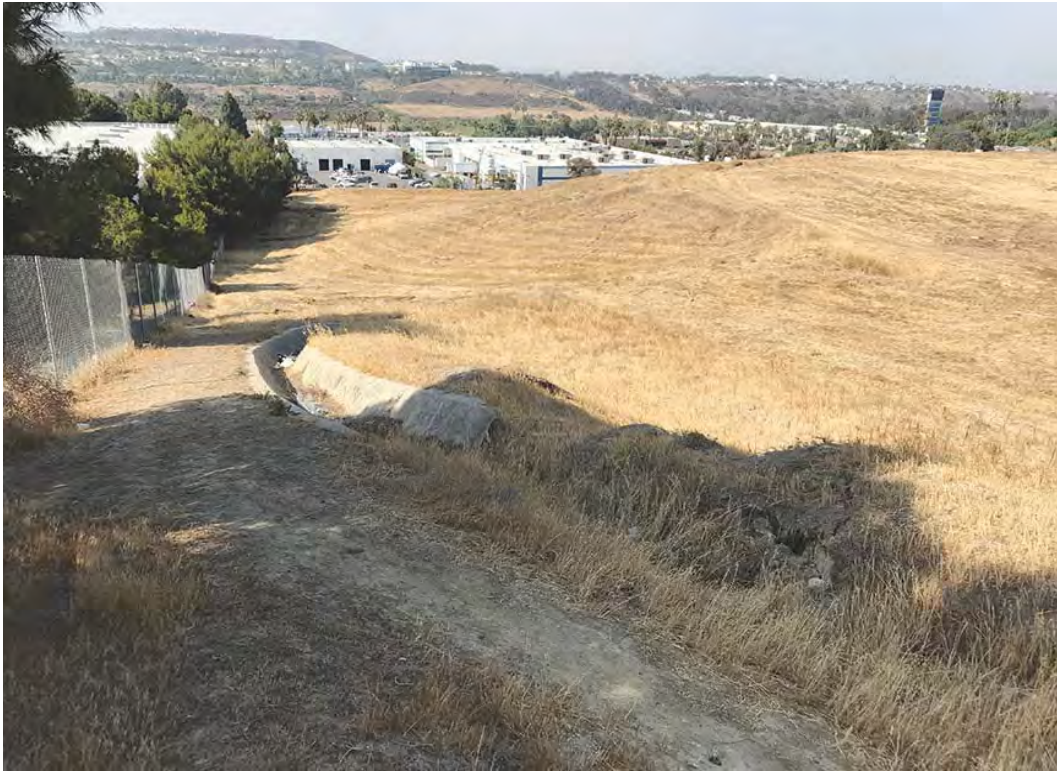
1) View of the concrete drainage in the northwest portion of the Site.
