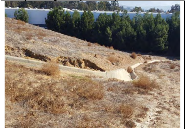
10. Stormwater channel on the central portion of the subject property with the east-adjacent building beyond.
