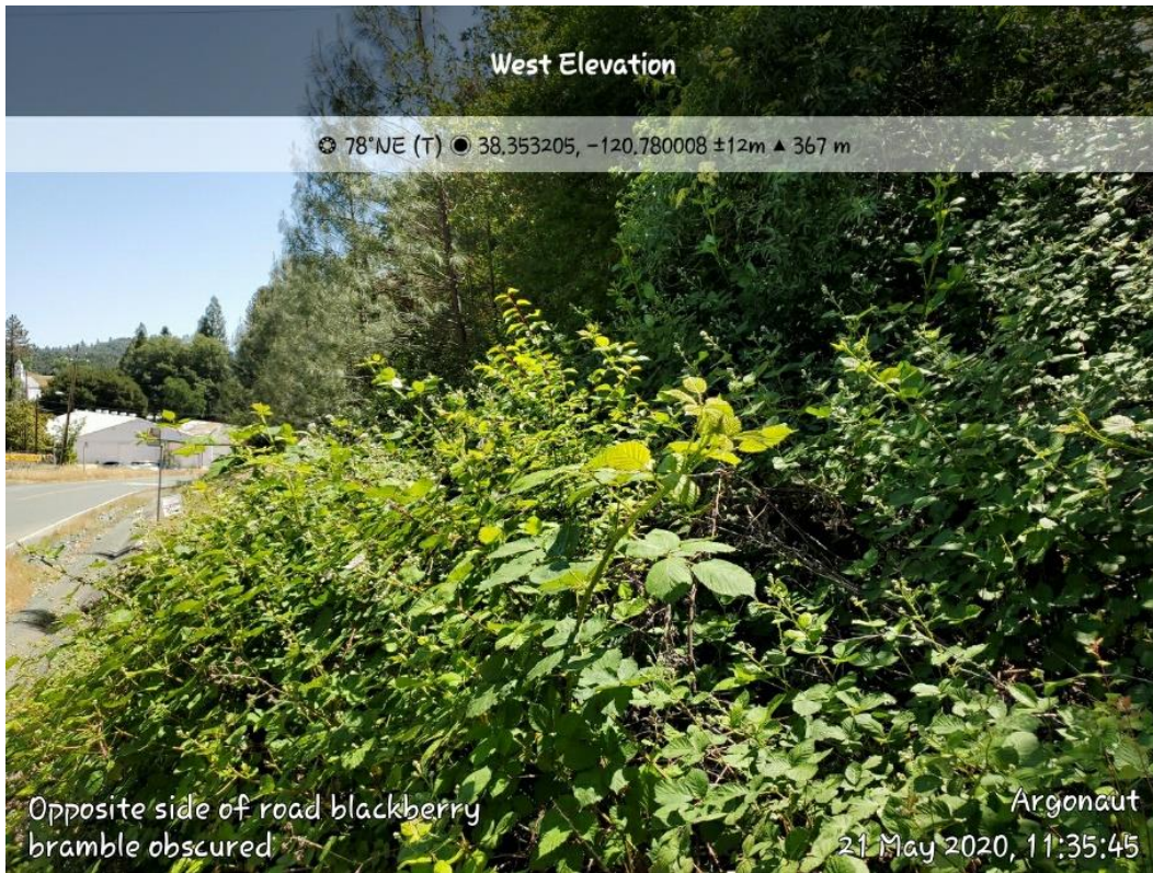
Figure 11. Blackberry Bramble growing across Sutter Street near retaining wall
