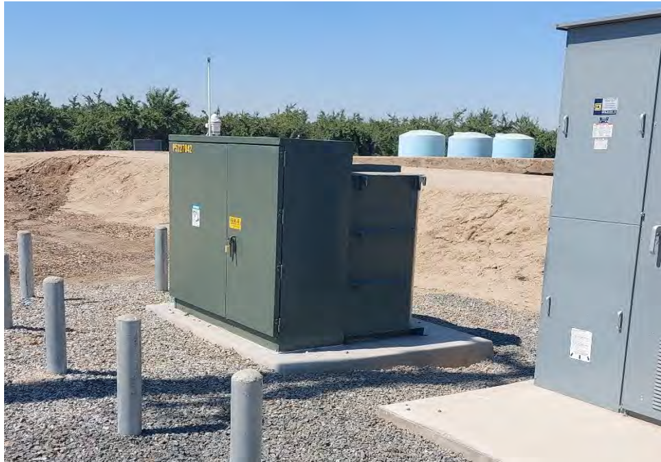
Photograph 3: Electrical transformers on top of concrete platform and gravel bed observed looking southwest, located west of Road 89, and south of north property boundary near canal, and east of water storage pond.
