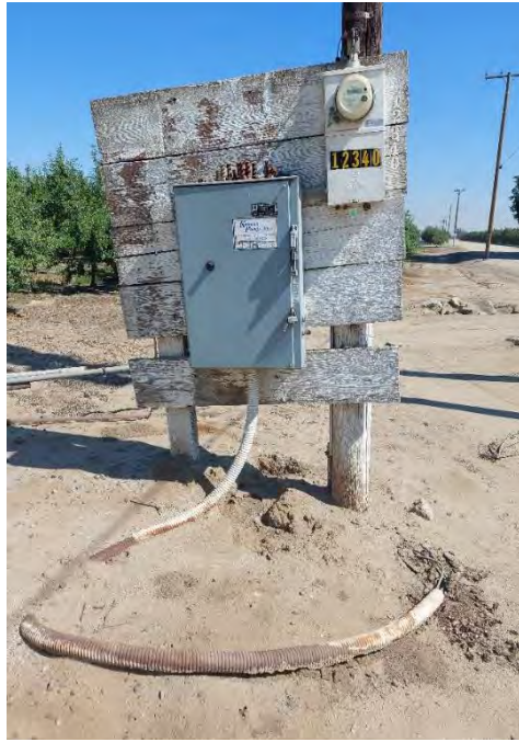
Photograph 1: Abandoned power station, observed looking north towards northern property boundary along canal. Located west of Road 89.
