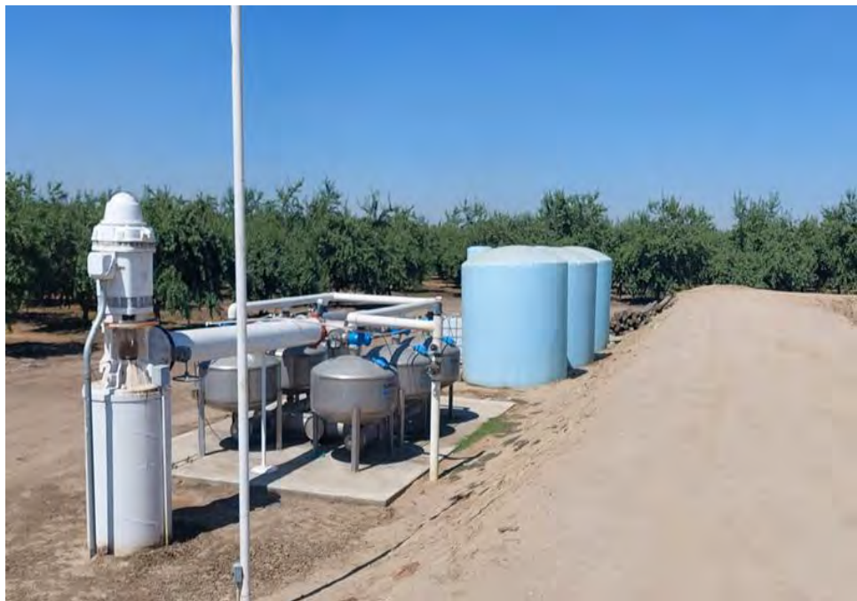
Photograph 4: View of filtration system located south of water storage pond, consisting of six filtration media tanks, and pump/pipe network. Located next to three approximately 2,000-gallon tanks and 250-gallon WM2 Concentrate Tote.
