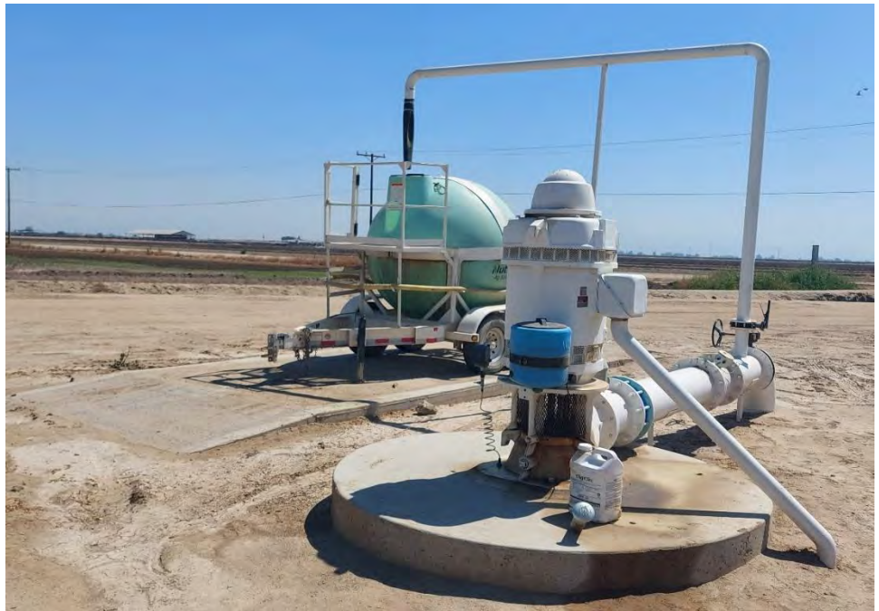
Photograph 6: View of an approximately 1,000-gallon water AST located south of northern property boundary and north of pond area.
