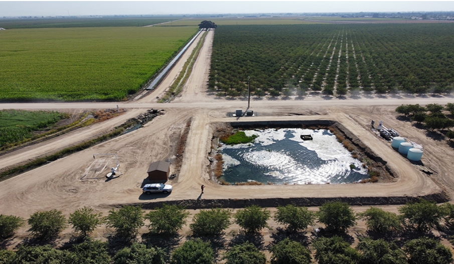
Photograph 7: Bird's eye view of the retention basin, southwest of road 89 and modoc ditch.
