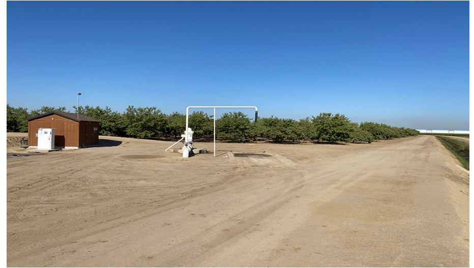
Photograph 8: Pump house at northern boundary of project site.
