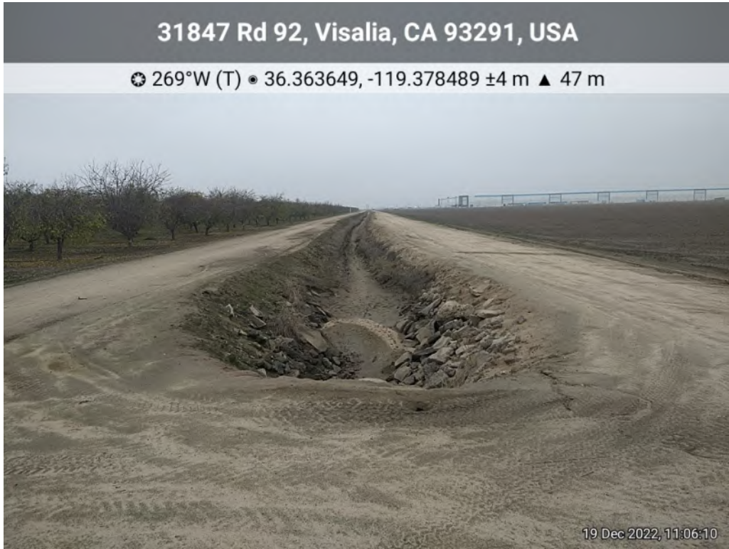
Photo 11. View of Modoc Ditch from culverted area under bare ground, facing west.
