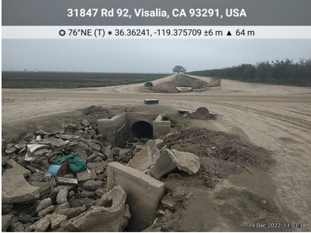
Photo 10. View of rip-rap, culvert under bare ground, and Modoc Ditch, facing east.
