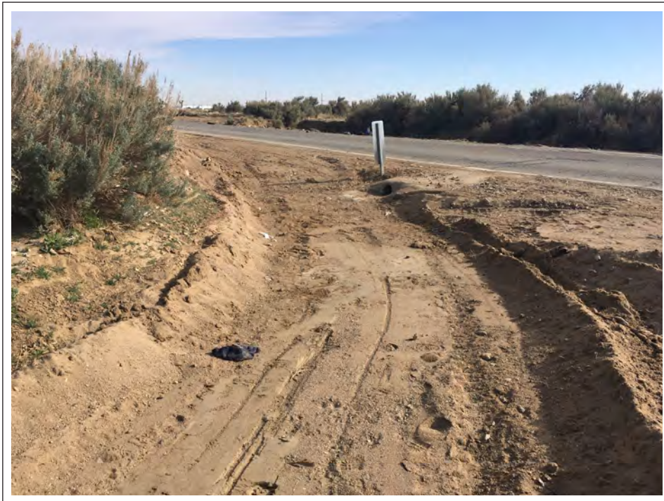
Photo Location 6, facing downstream. March 17, 2022. View of conditions where stream channel flows toward 8th Street along eastern site boundary. Note that road shoulder is graded to allow water to flow off road into channel. Small culvert is evident that allows water to drain eastward under 8th Street.
