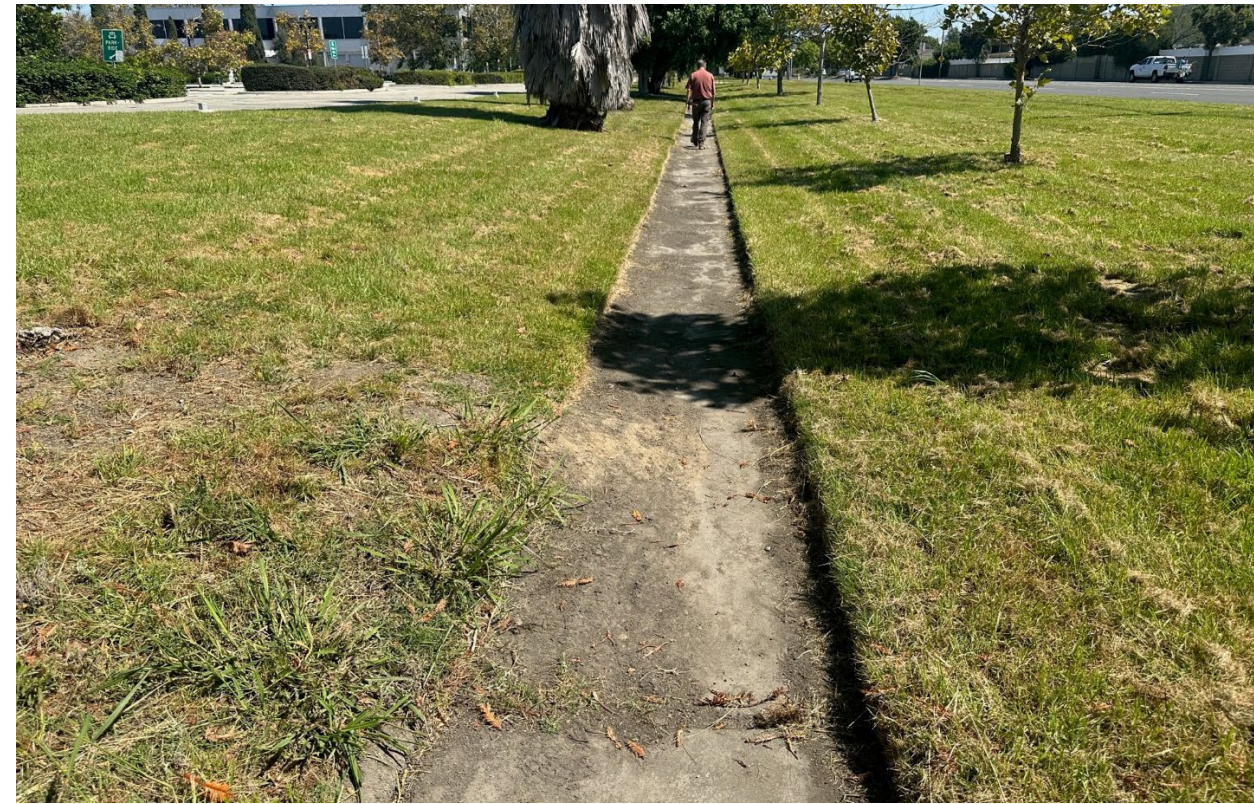
Photograph 2: View of shallow concrete ditch looking east immediately east of outfall shown in Photograph 4.
