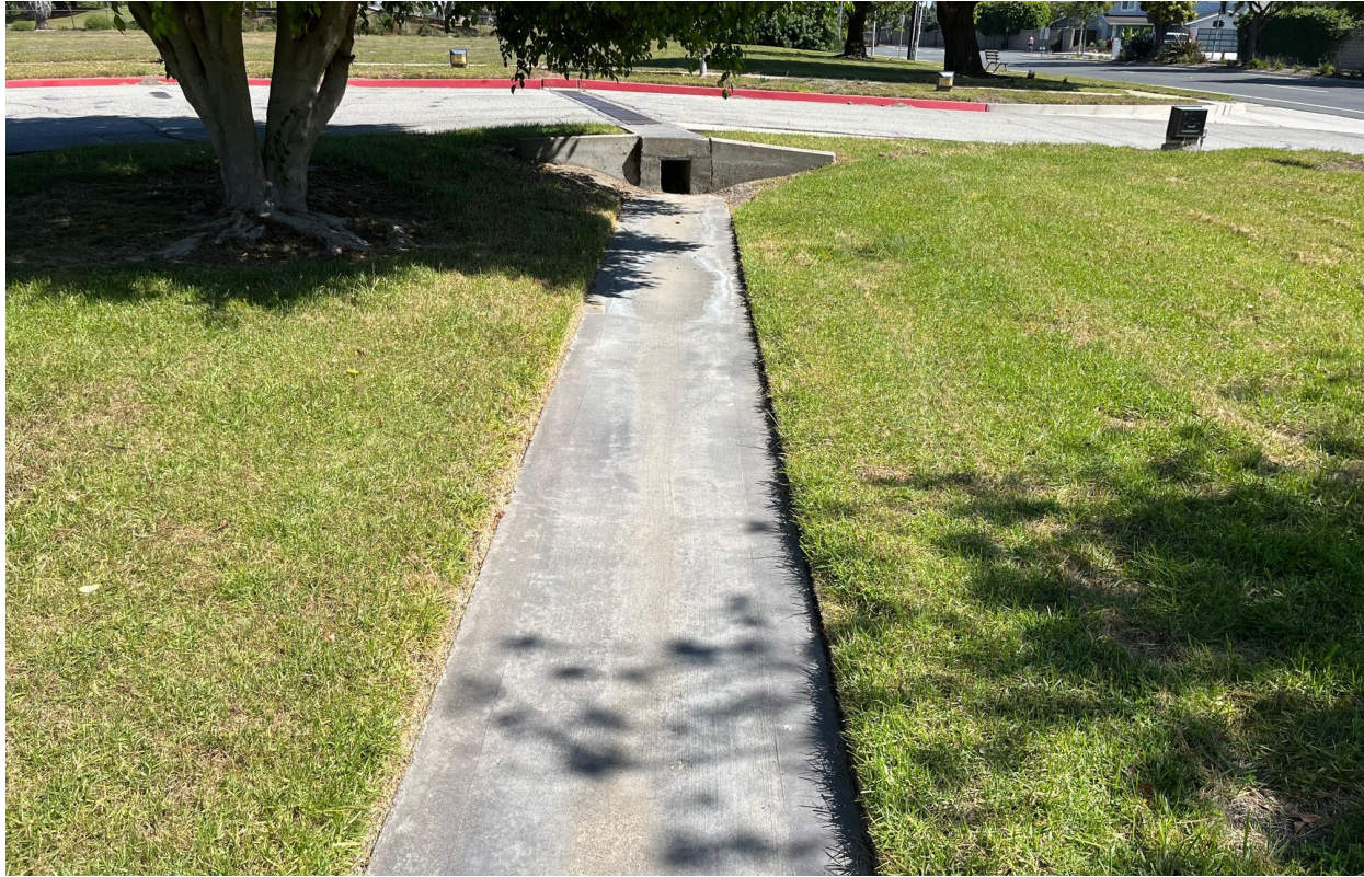
Photograph 5: View of shallow concrete ditch looking east showing no sediment accumulation near the inlet structure at terminus of ditch.
