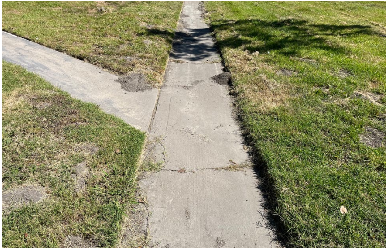
Photograph 1: View of shallow clean concrete ditch looking east immediately east of outfall shown in Photograph 4.
