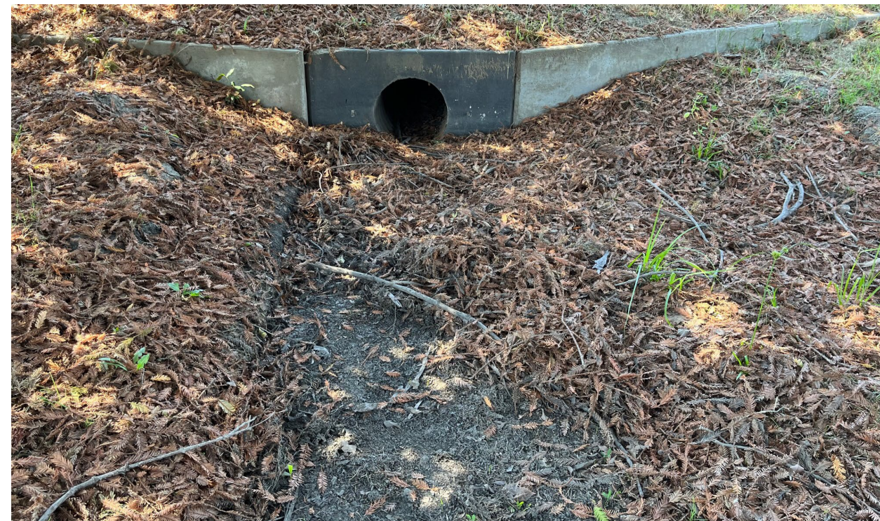
Photograph 4: View concrete ditch at outfall showing shallow sediment accumulation and leaf litter from overhanging ornamental coast redwood.
