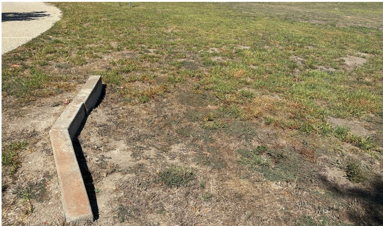
Photograph 7: View of outfall that is fully blocked with sediment east of road shown in Photographs 6 above and Photograph 8.
