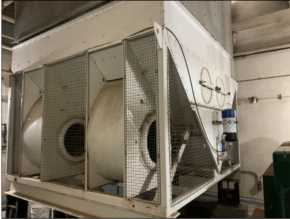
Photo 39: View of mechanical room.
