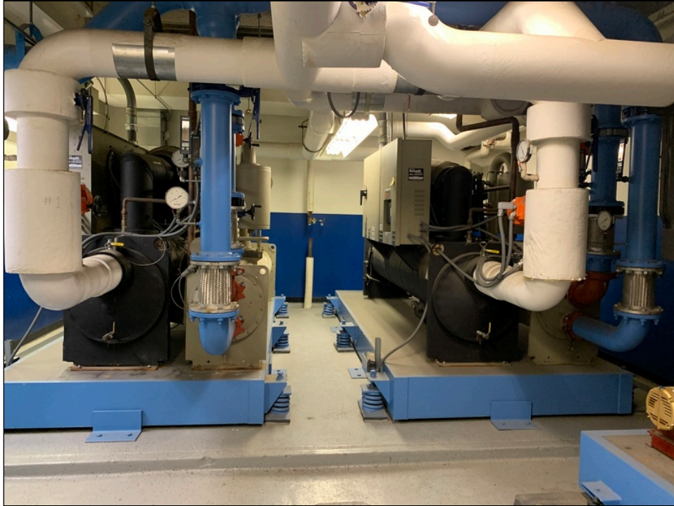
Photo 40: View of chiller room.
