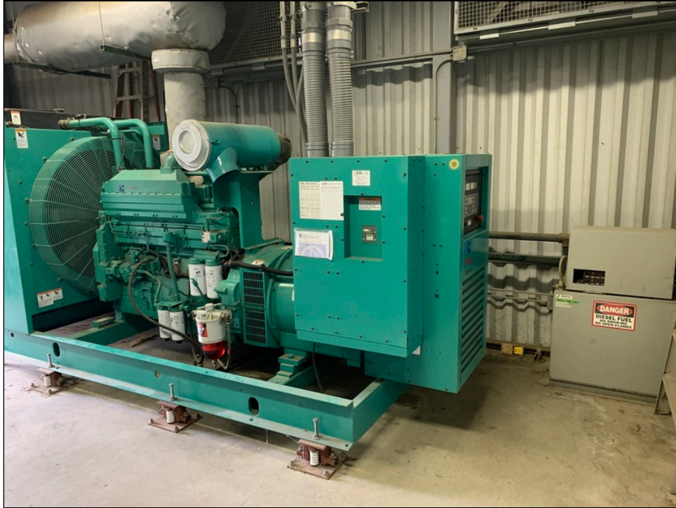
Photo 36: View of emergency power generator.
