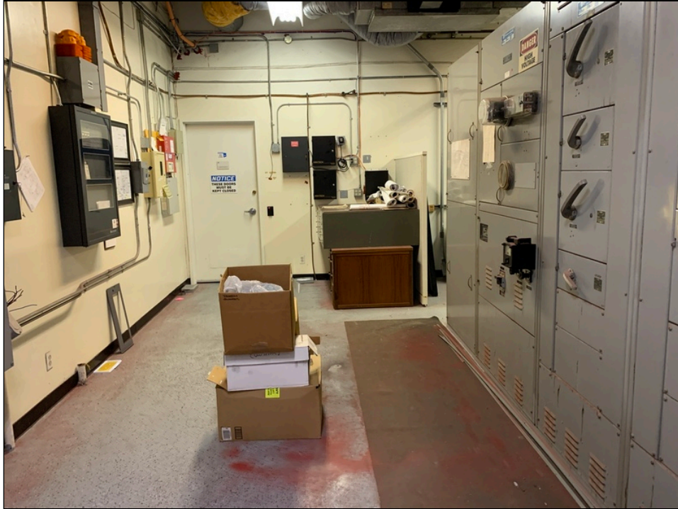
Photo 34: View of electrical room.
