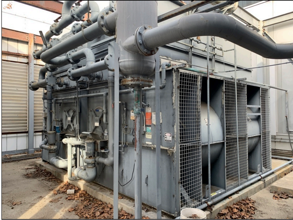
Photo 19: View of cooling equipment within the enclosure west of the subject structure.
