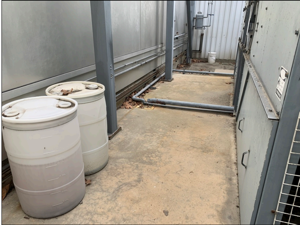
Photo 20: View of 55-gallon drums and drain.
