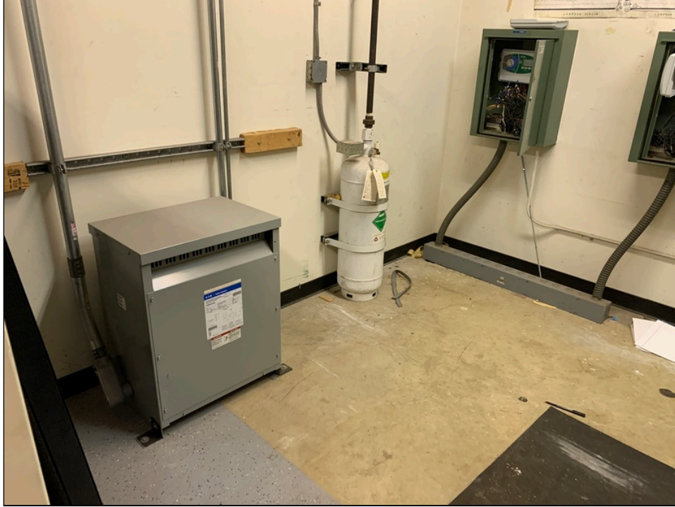
Photo 35: Representative view of dry-type transformer.
