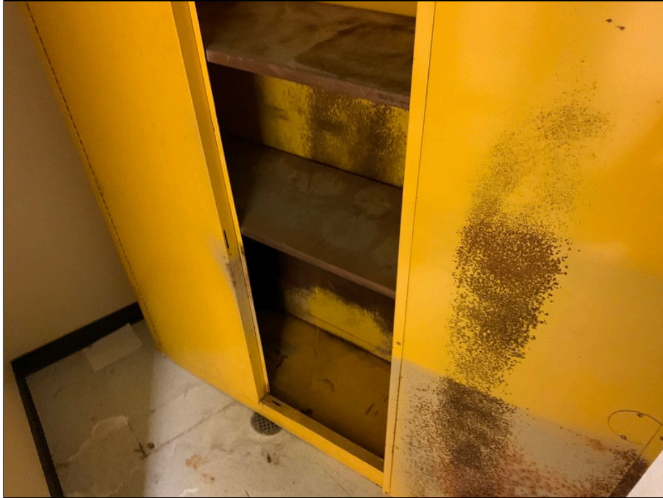
Photo 44: View of empty flammable material cabinet.
