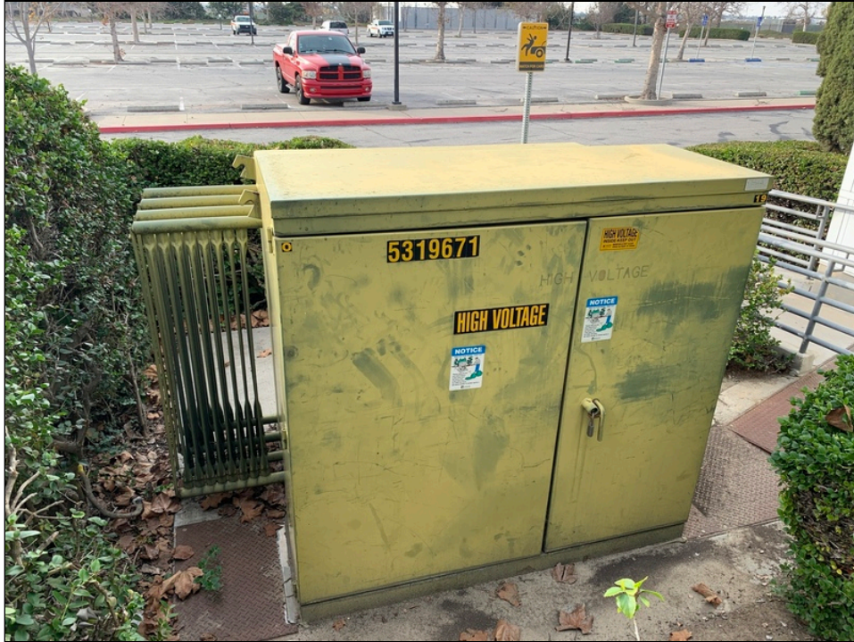
Photo 18: View of pad-mounted electrical transformer.
