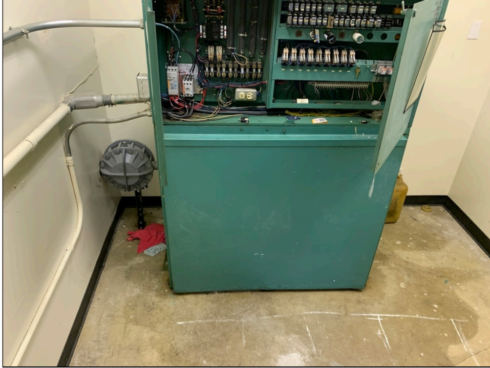
Photo 37: View of elevator equipment room.
