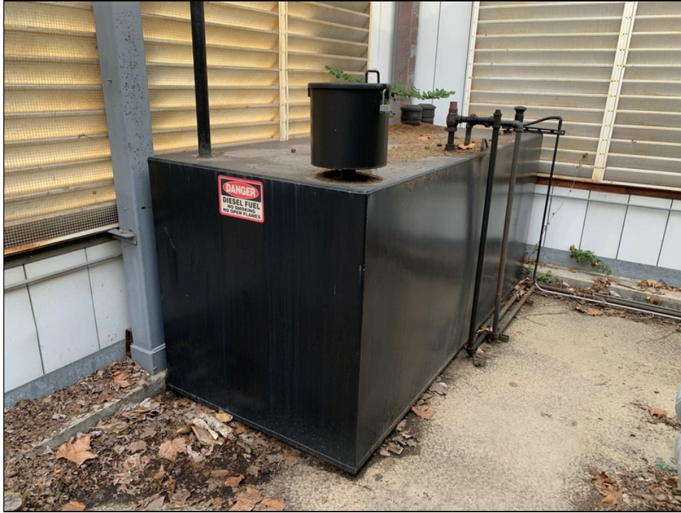
Photo 21: View of diesel AST.
