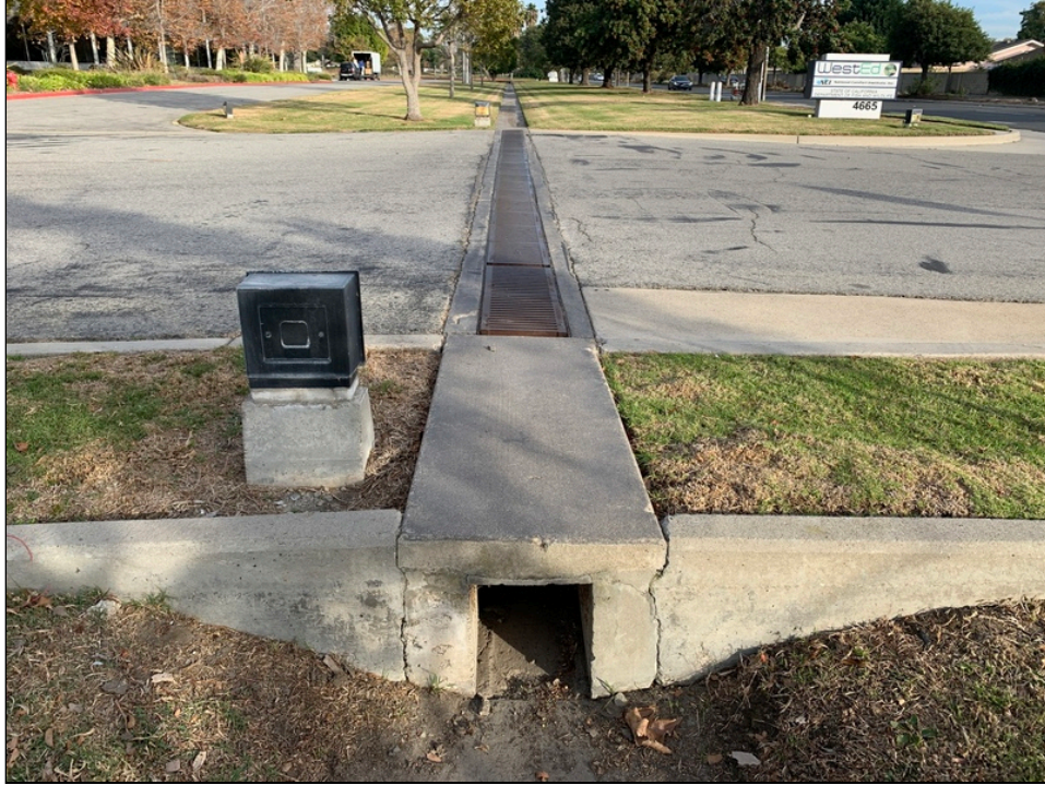
Photo 25: Representative view of trench drain.
