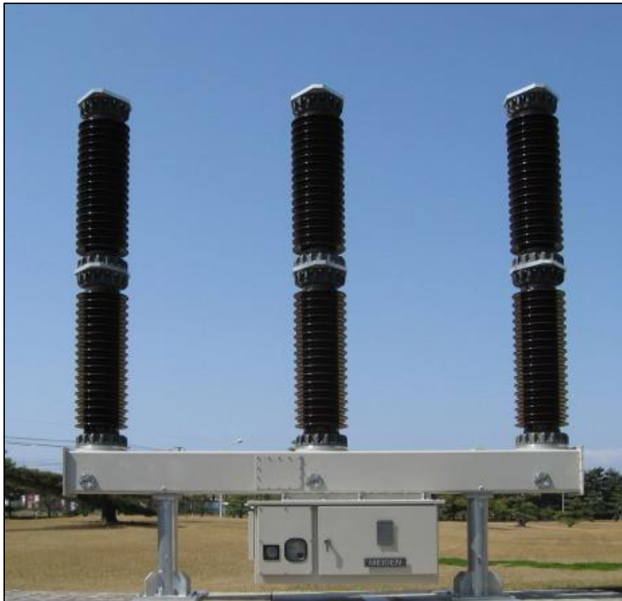
145KV Meiden vacuum breaker
