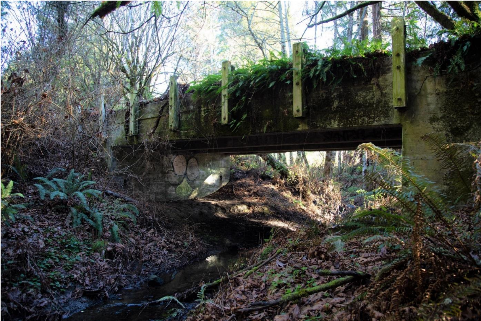
Figure 4. Old Ward Creek Bridge, approximately 100 feet downstream of existing culvert and SR 36
