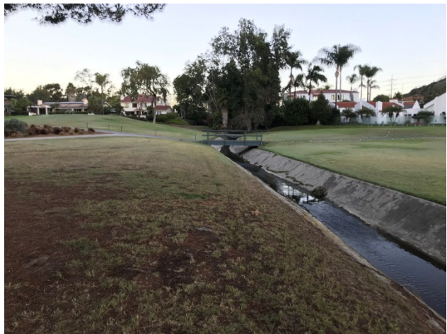
Photo of concrete channel portion of Drainage A, looking south from just south of Alga Road crossing.
