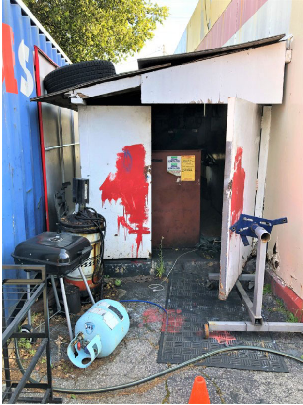
Photo 1. Hazardous waste storage on backside (northwest) of onsite building – Shed and secondary containment for waste oil AST, 20-gallon mobile waste oil drain tank, and stained concrete in poor condition. Photograph taken March 16, 2021.
