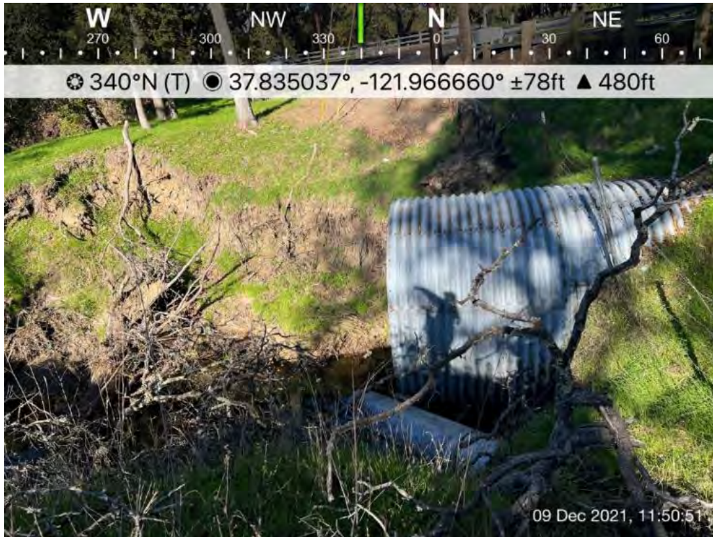
Photograph 1: View of culvert that conveys East Branch Green Valley Creek beneath Diablo Road.
