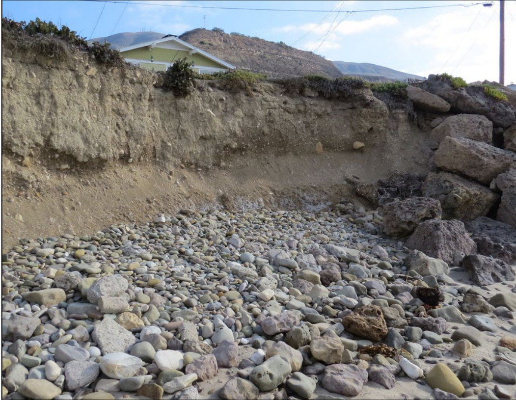
Figure 16. Eroding bluff immediately downcoast from abutment that is fronted by a cobble berm but no riprap.
