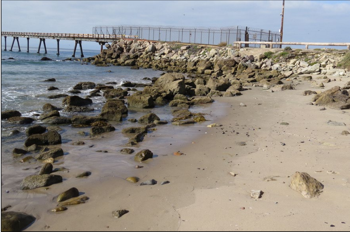
Figure 15. October 2, 2022, view towards the abutment and causeway showing riprap that has migrated east or downcoast since original emplacement in 1959.
