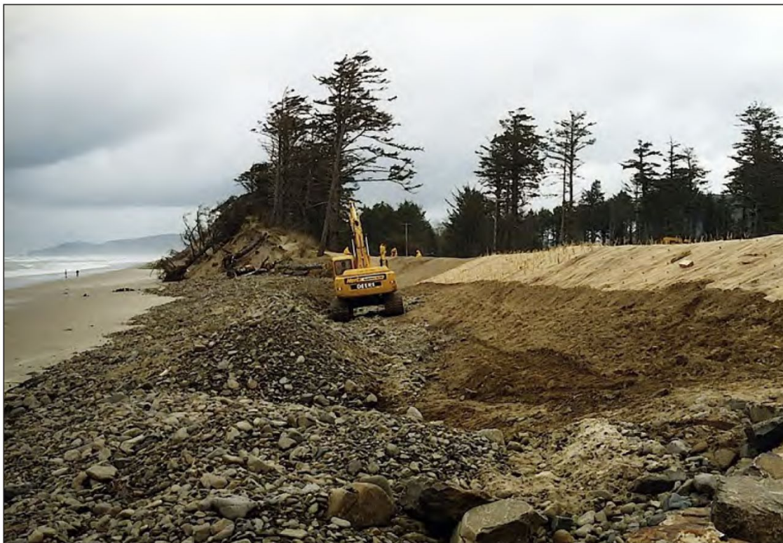
Figure 21. Cape Lookout State Park cobble berm under construction (from Komar and Allan, 2009)
