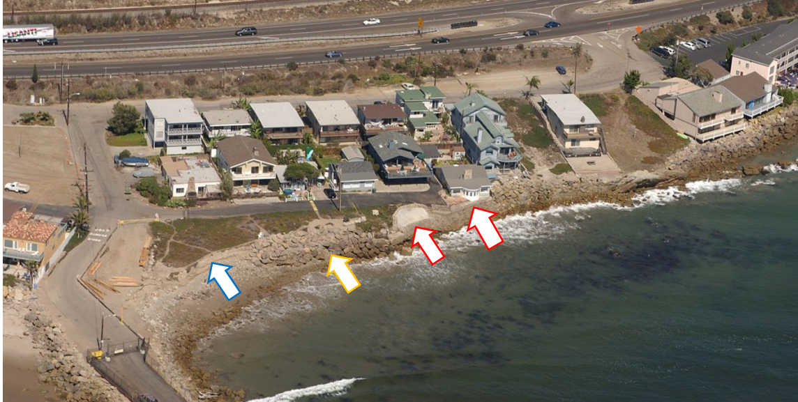
Figure 13. 2002 photograph showing two concrete seawalls at downcoast end of SCC parcel (red arrows) and riprap now added upcoast of the seawalls (orange arrow). The low bluff is now fronted with a scarp along its entire western section (blue arrow) (California Coastal Records Project – Kenneth and Gabrielle Adelman).
