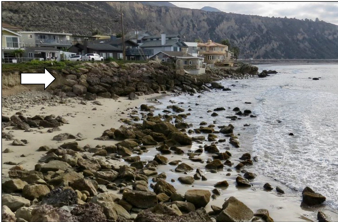
Figure 30. Riprap (arrow) protecting Breakers Way and downcoast homes and remnants of original 1959 riprap scattered along the shoreline.
