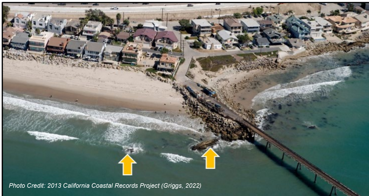
Figure 2-5. Nearshore Bedrock Outcrops Forming Punta Gorda Adjacent to Updrift Side of Abutment
