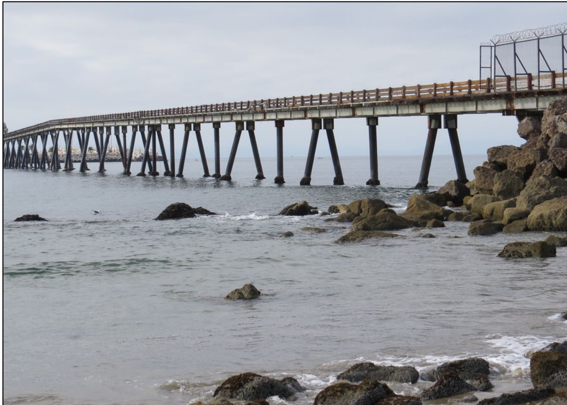
Figure 29. View of the causeway from downcoast showing wide spacing and small diameter of pilings.
