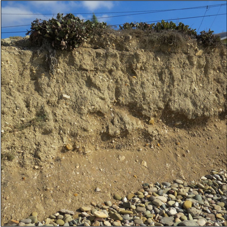
Figure 42. Eroding coastal bluff immediately east of the abutment.
